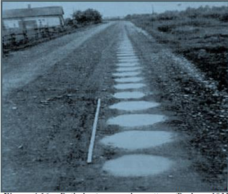
Figure 2-3 regular potholes on gravel roads (source [23])
