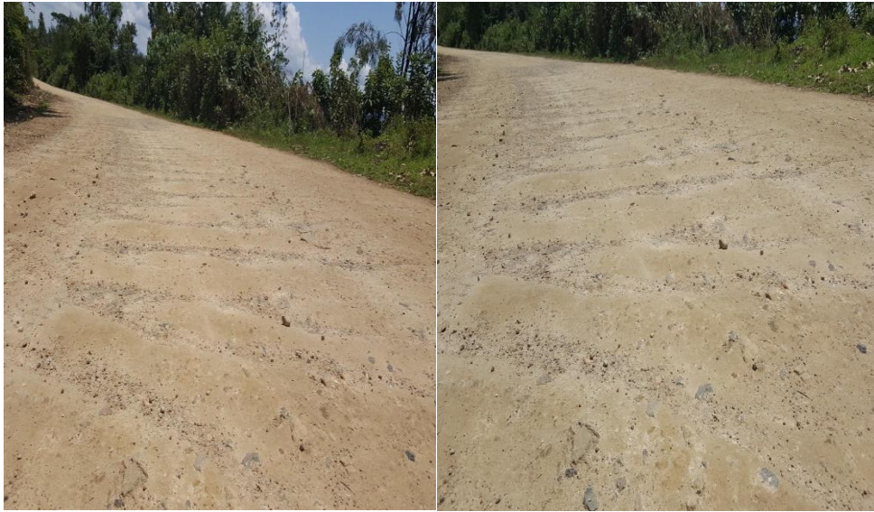
Figure 4-8 Failure observed on road corrugation
