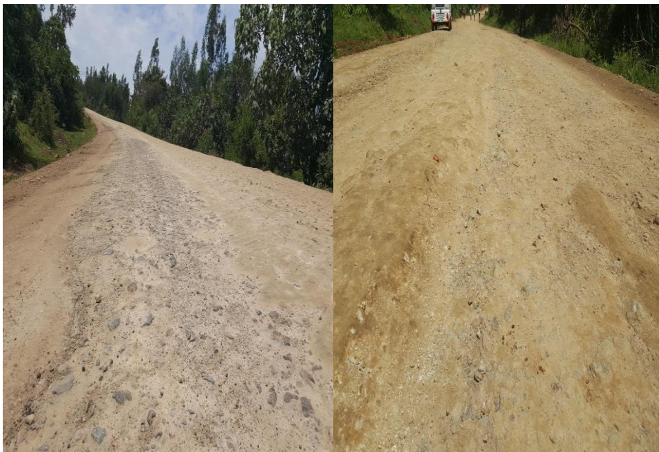
Figure 4-9 Failure observed on road raveling
