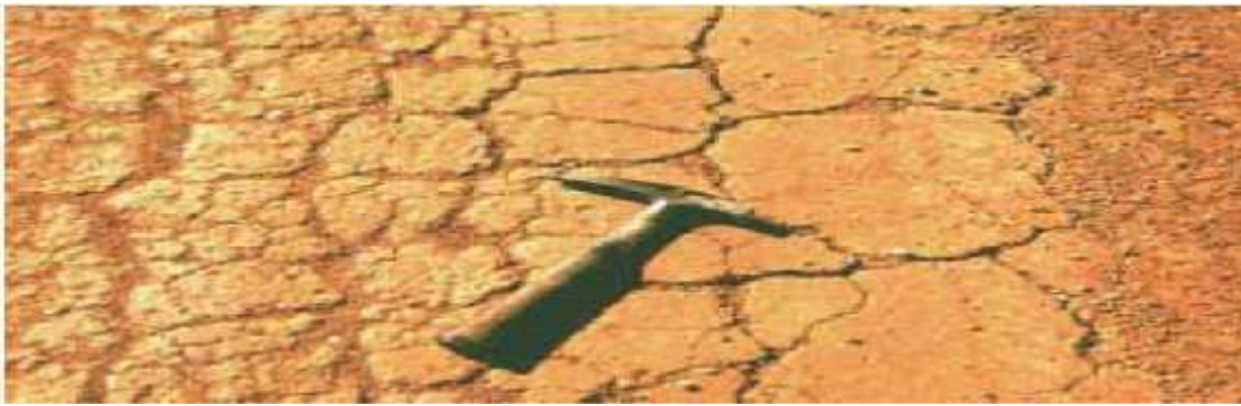
Figure 2-6 cracks on unpaved roads (source [23])
