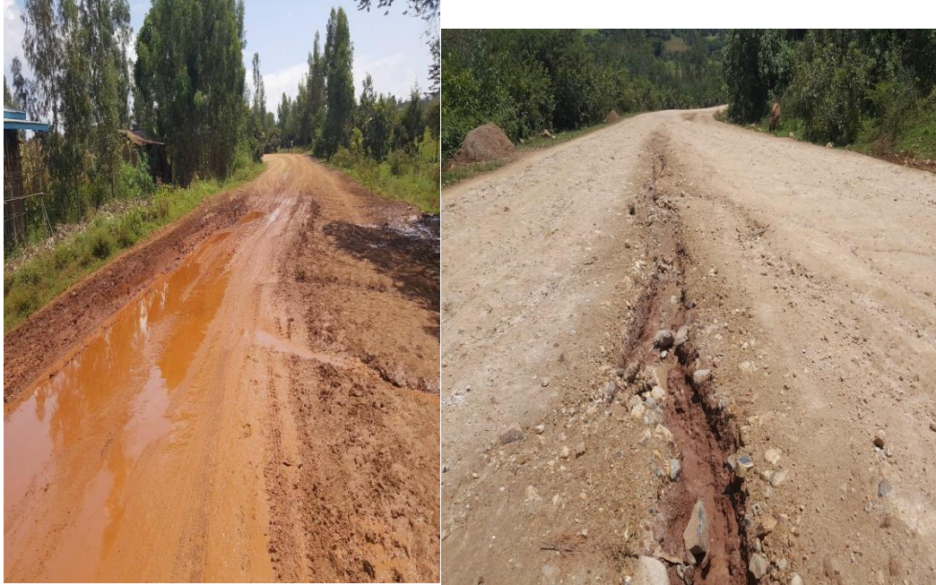
Figure 4-10 Failure observed on the road: slipperiness and impassibility
