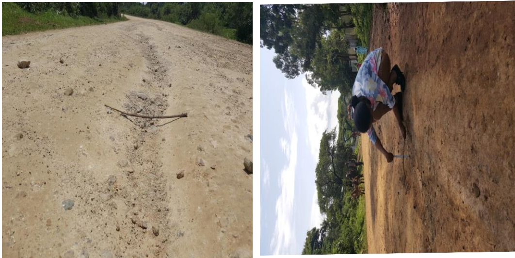
Figure 4-6 Failures observed on the road: pothole
