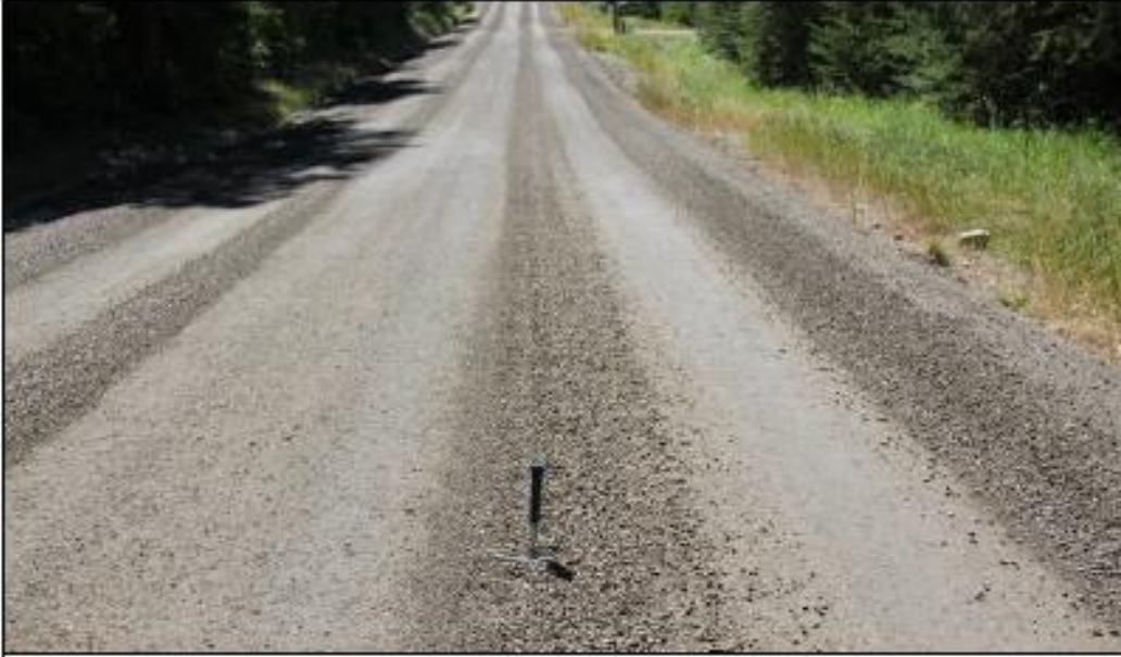
Figure 2-7 raveling on unpaved roads (source: [18])
