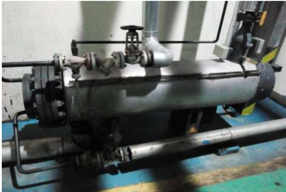
Figure 1.2 Existing shell and tube heat exchanger in Dashen Brewery Industry
