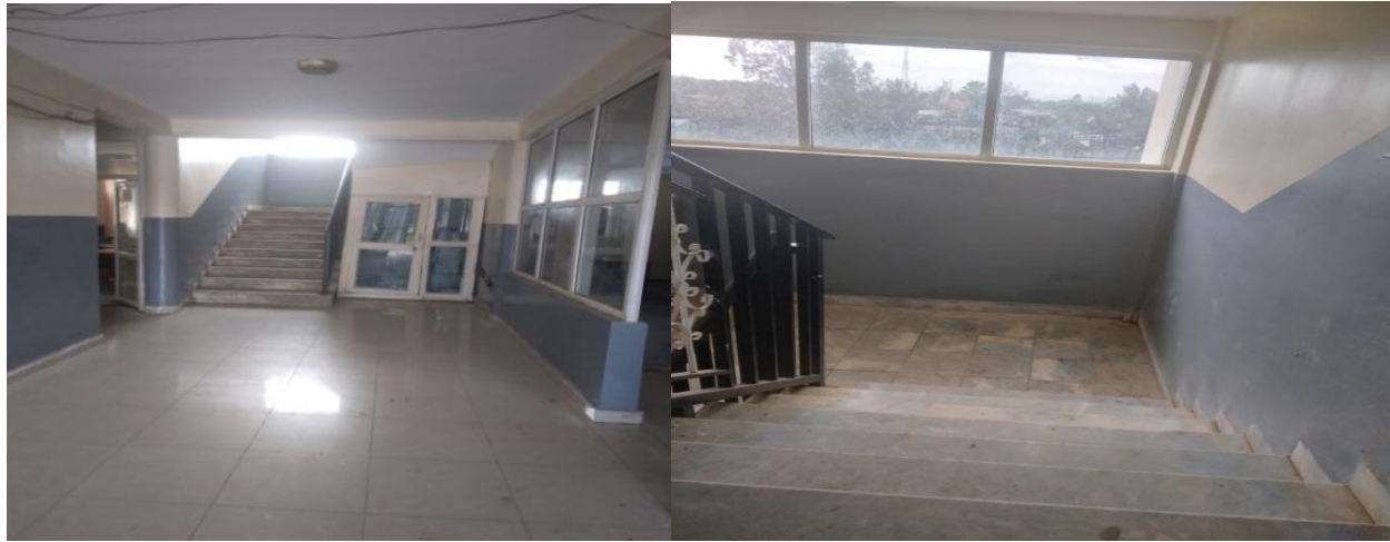
Figure 4.12. Southwest Shewa zone administration building natural lighting and ventilation (Source by Author, 2023)
