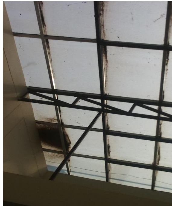
Picture 8 Leakage underside of roof cover
