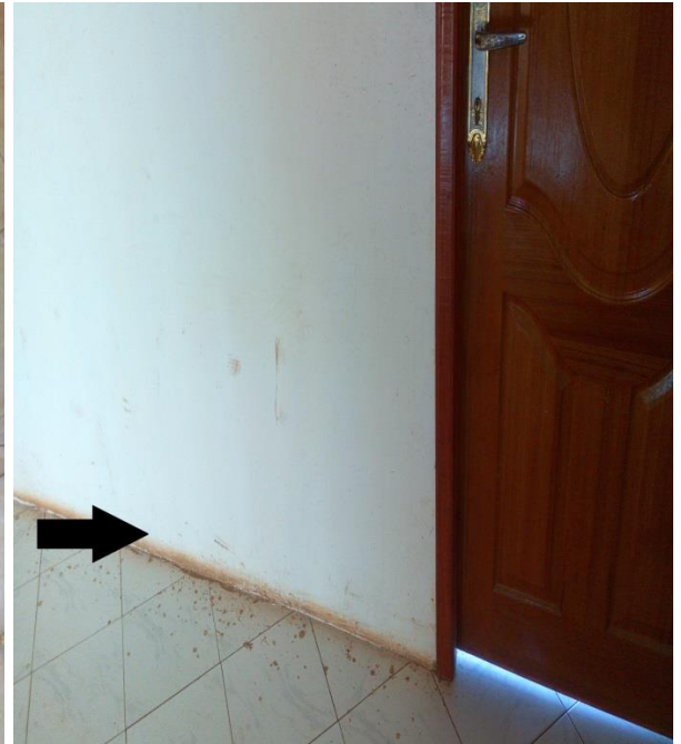
picture 12 Missing skirting
