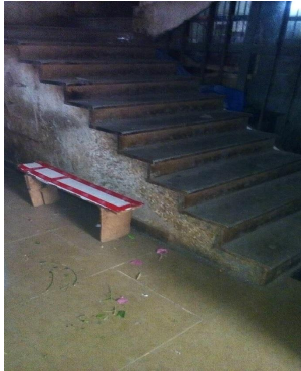
Picture 6 Missing handrail on both sides
