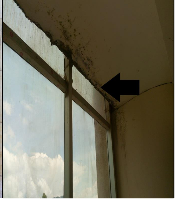
Picture 10 Water seepage through windows
