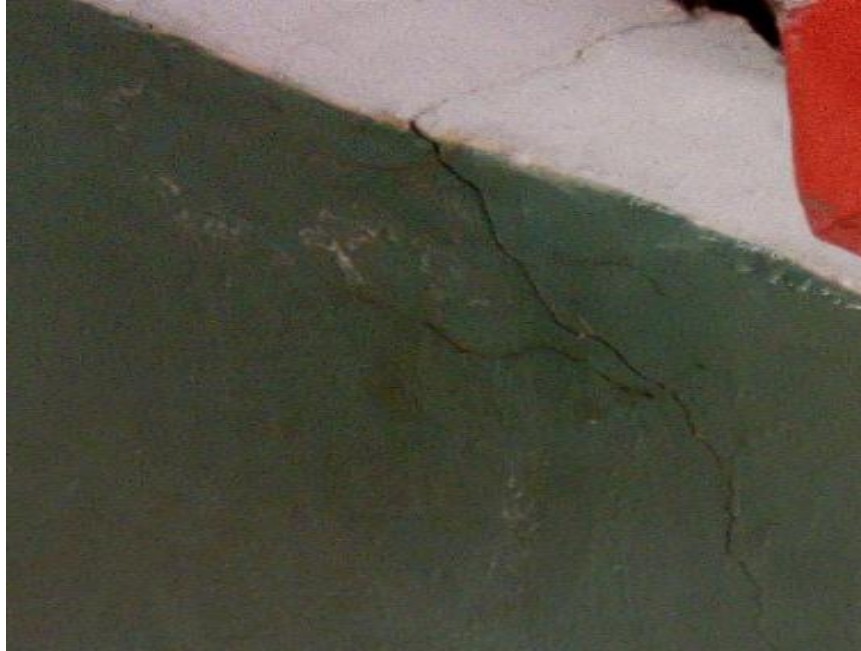
Fig. 4.1 plastering crack (observed on sample building of building P004)
