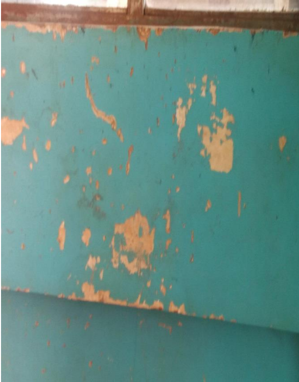
Picture 1 Peeling off paint
