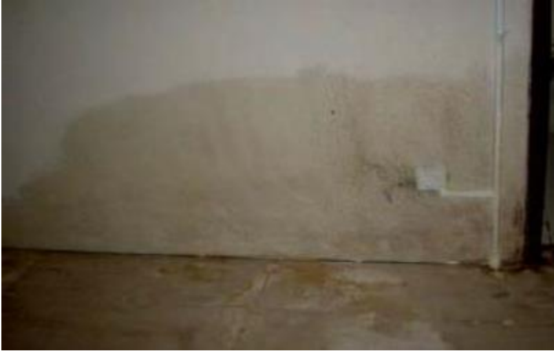
Figure 2.1. Rising Dampness (Bakri, 2014)
