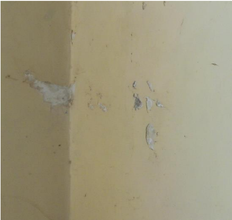
Figure 4.4 Paint peeling on internal wall (observed on sample building 009)
