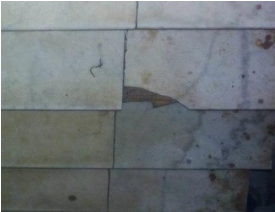
Figure 4.6 broken floor tiles (observed at sample building P006)
