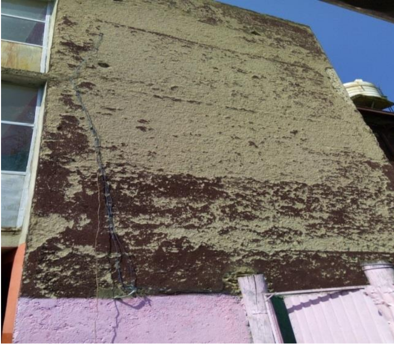
Figure 4.3 Paint peeling on external façade wall (observed on sample building 004)
