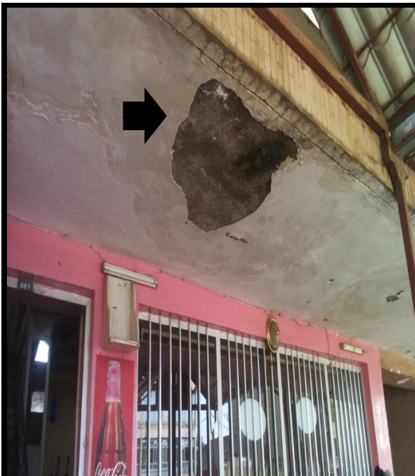
Picture 7 Detachment of plastering
