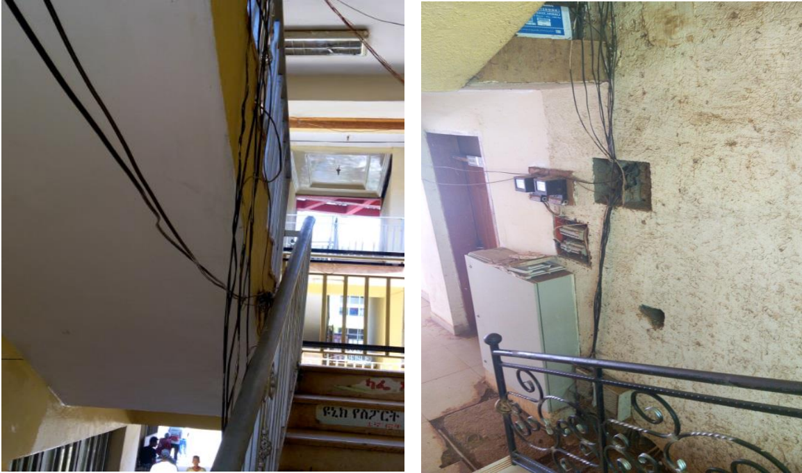
Figure 4.7 exposed electrical wiring (observed on buildings P003 and P010)
