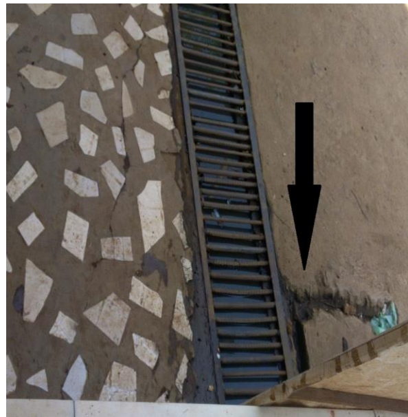
Picture 4 Defective wastewater drainage system
