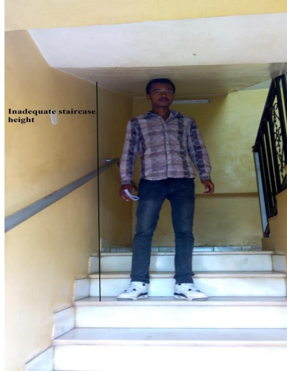
Picture 2 Inadequate height of staircase
