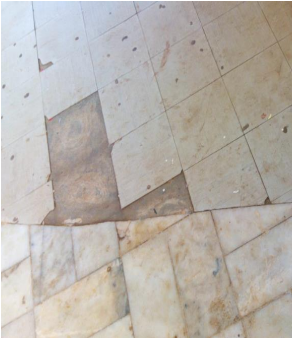
Picture 11 Broken floor tiles
