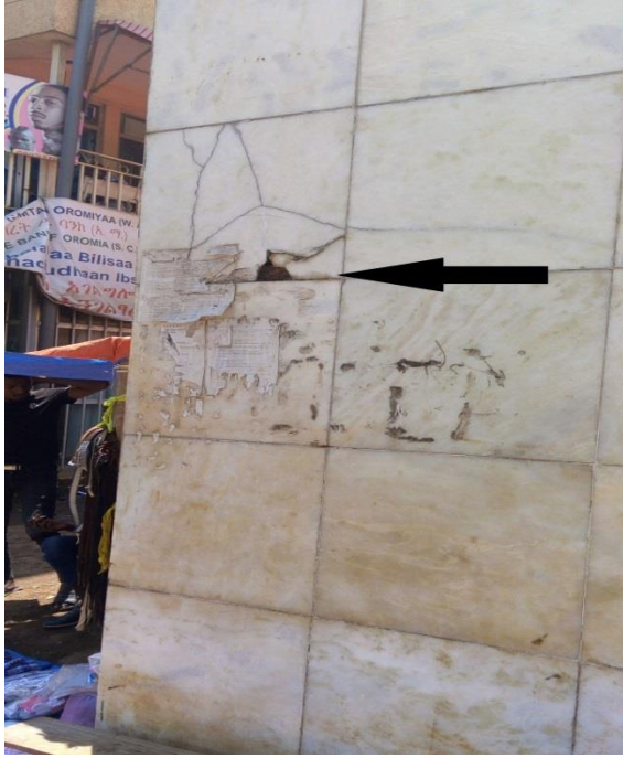
Picture 9 Broken ceramic wall tiles
