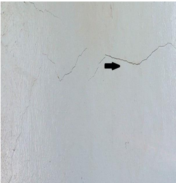
Picture 3 Plastering cracks
