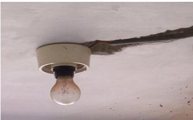
Figure 4.8 Defective electrical wiring due to poor workmanship (observed on building P012)
