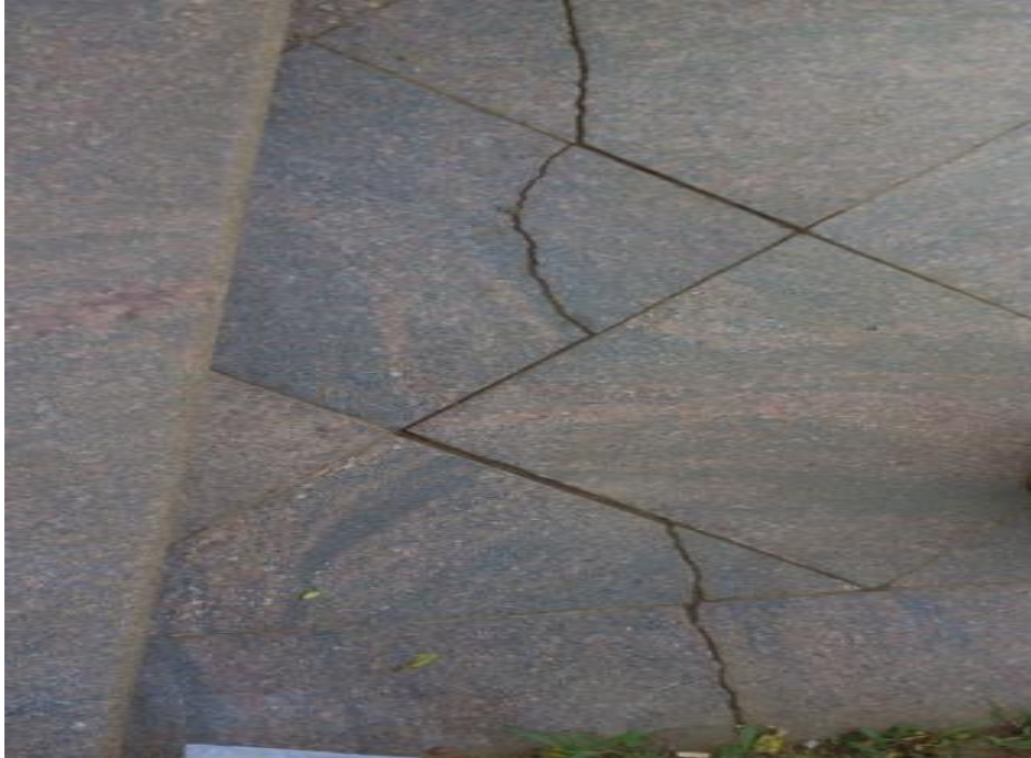
Figure 4.5 Cracked floor tiles (observed at sample building P006)
