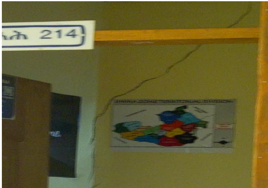
Fig. 4.2 plastering crack (observed on sample building of building P008)
