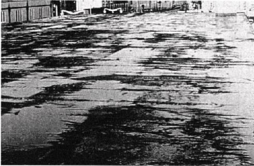
Figure 2.3 Ponding on flat roof—a state typical of many flat roofs (W. H. Ransom)
