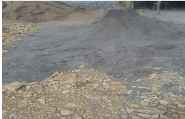
Figure 4.3 Improper placing of coarse aggregates
