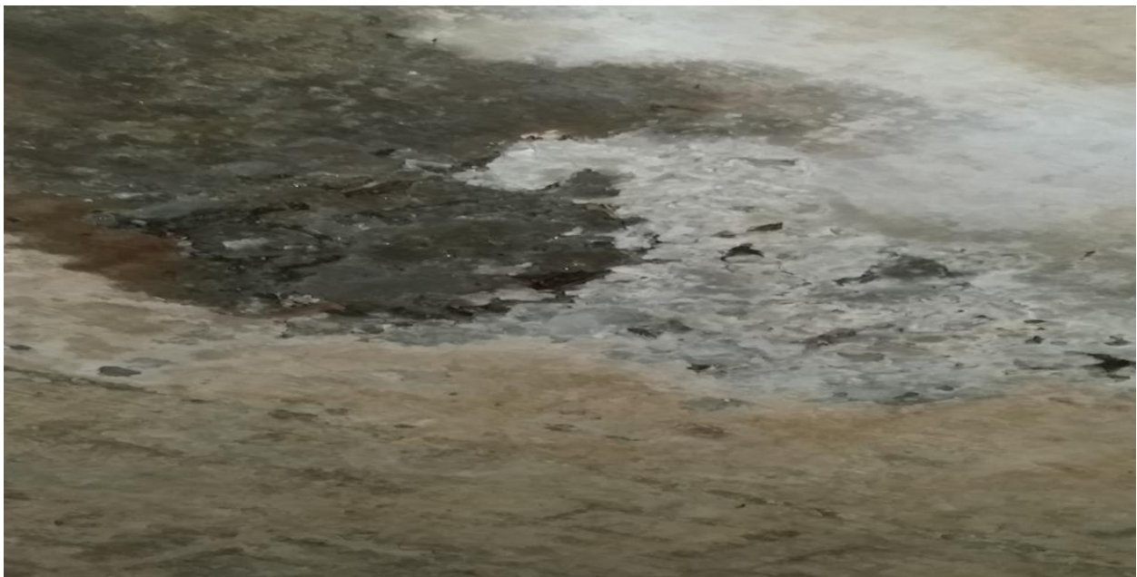
Figure 6 Segregation under the slab caused by over vibration compaction.
