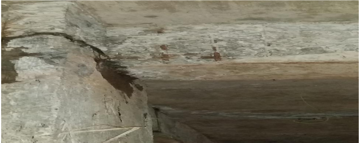
Figure 5 Uncovered reinforcing bar seen under the beam caused by poor (under vibration) compaction.
