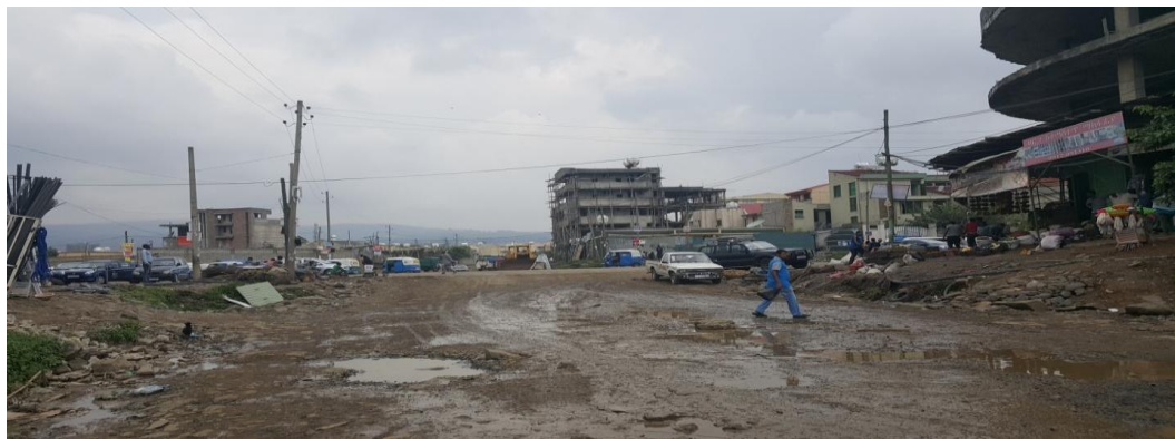
Figure 4.6: Yerergero school- CMC at st. Michael Church –Kotebewendyrad School Asphalt concrete road project.
