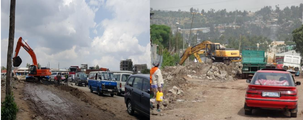
Figure 4.27 High traffic volumes and no road way sign available
