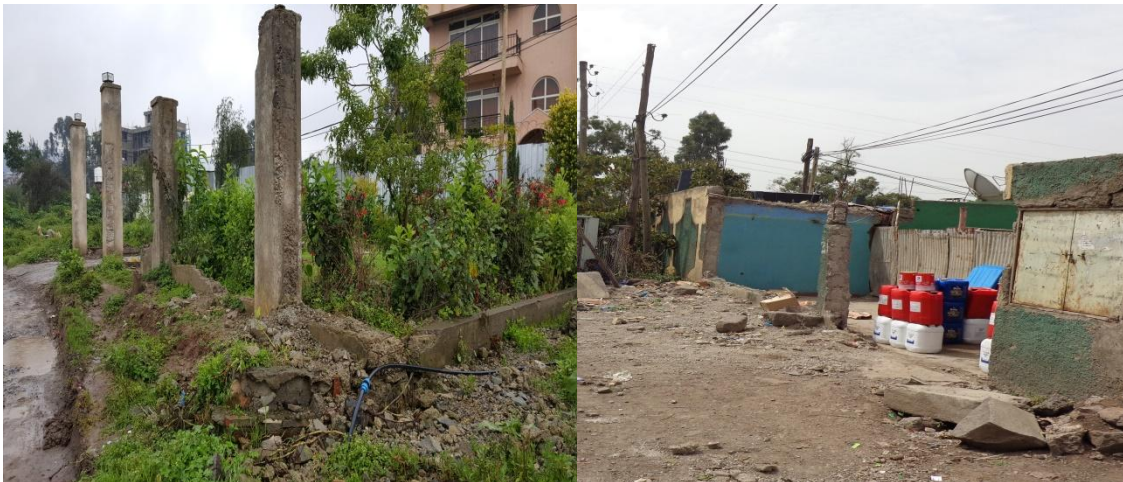
Figure 4.21:Partially demolished building on Cmckaralo junction and kadsico
