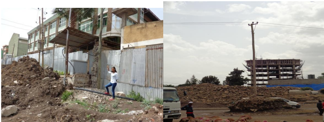
Figure 4.25: slow clearance of Electric pole and Tele wire box (Kadiskopaint factory – Crown Hotel, Meskel flower- Gazebo)
