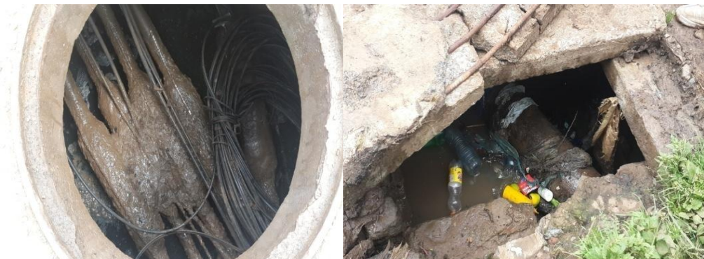
Figure 4.26: Bundles of underground optical fibers and copper cables at 0+420km which crosses the road project (2nd police station – kideste Mariam)
