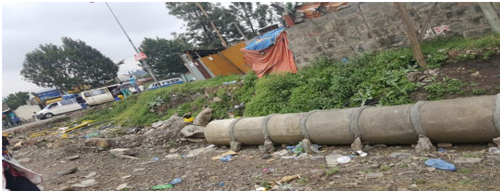
Figure 4.7: km4+600 DCI pipe not relocated by EEU junction work.
