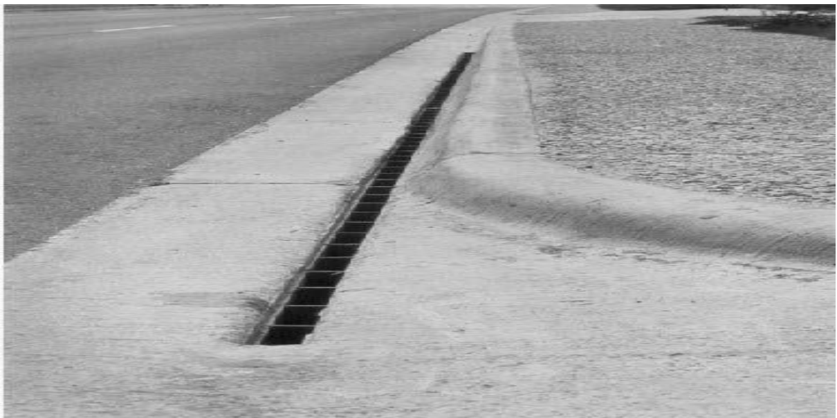
Figure 2.4 Slotted drain inlet at an intersection
