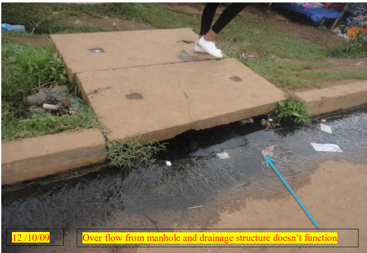
Figure 4.9 that drainage fills by debris (taken around bus station & feid roundabout)
