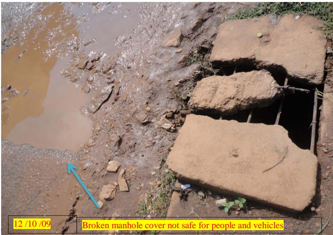
Figure 4.8 shows that manual cover damage and removed in front of total (source: field survey).
