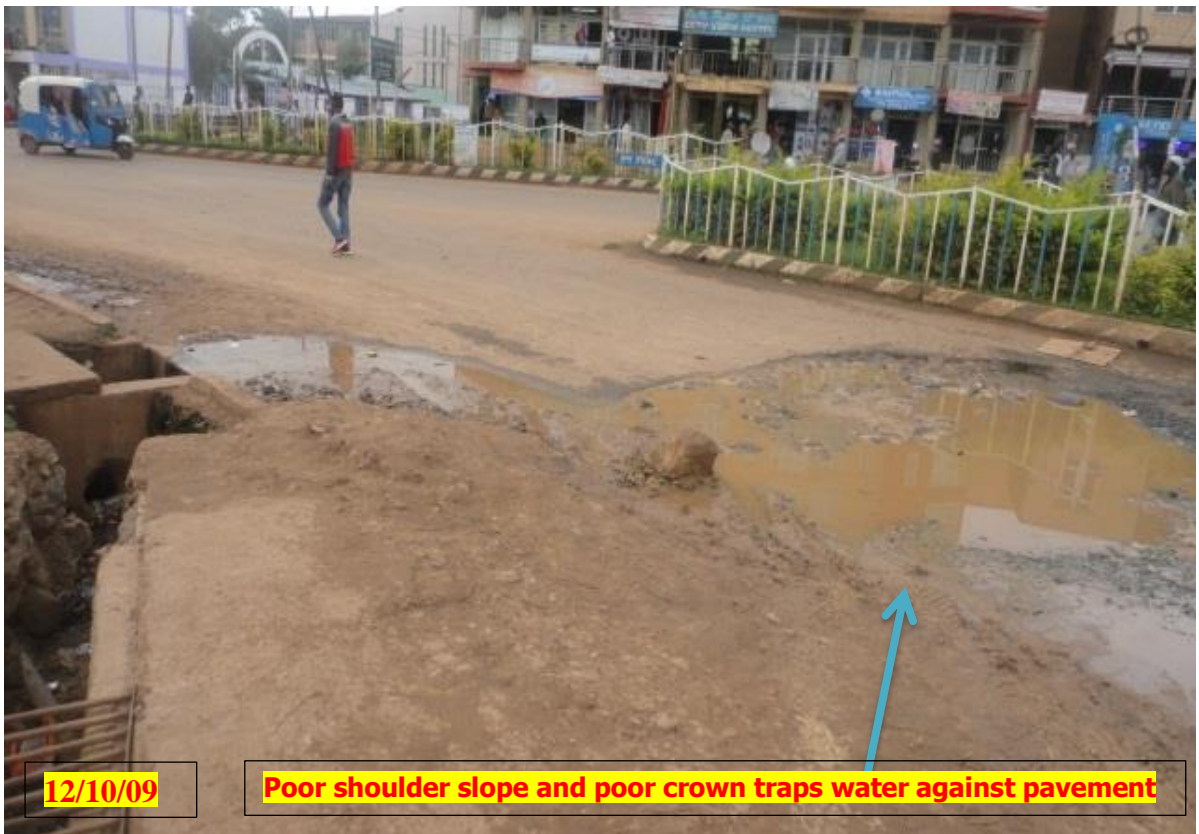
Figure 4.19 Formation of potholes due to Poor Drainage around genu hotel
