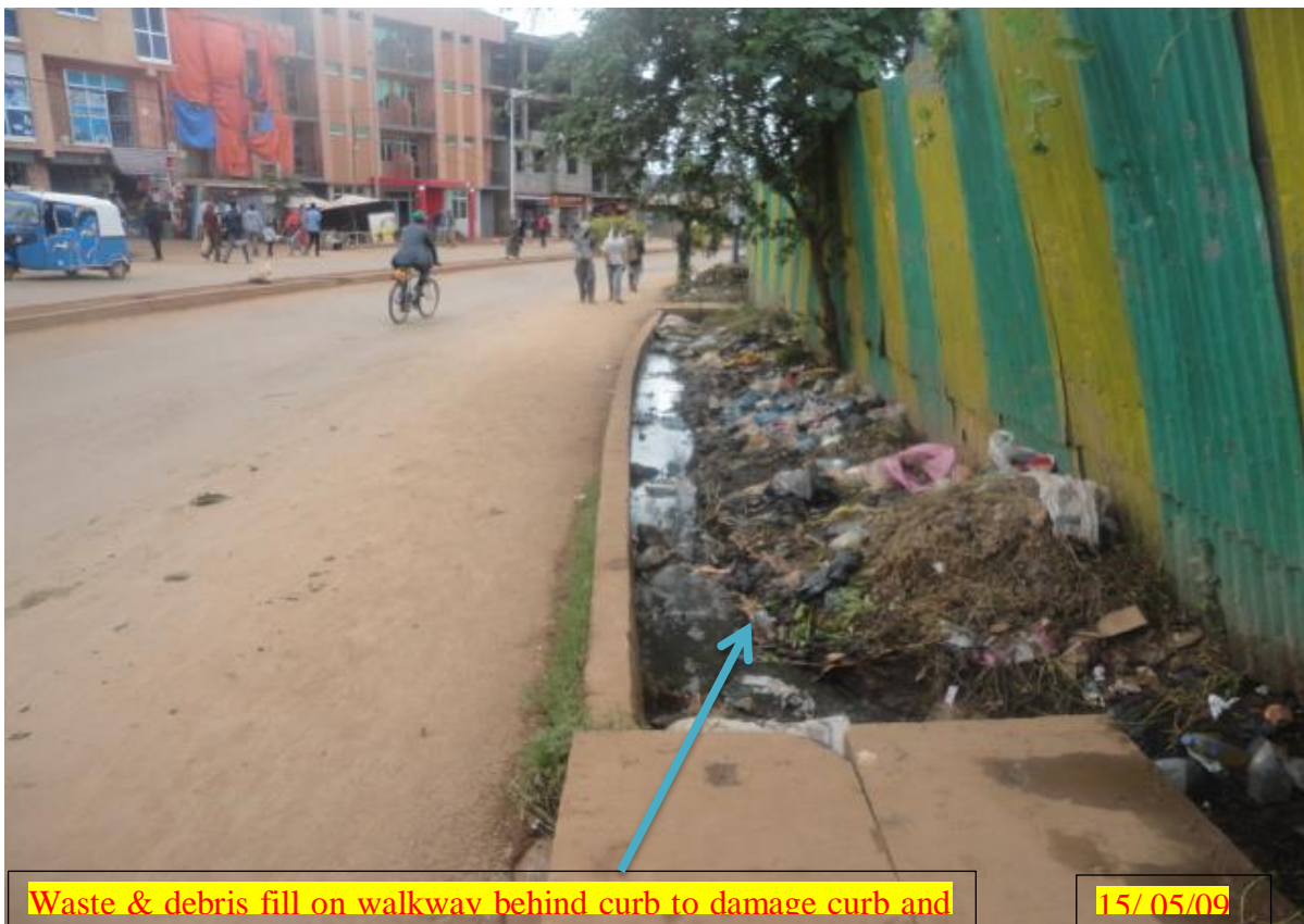
Figure 4.5 waste disposal on the drainage structure
