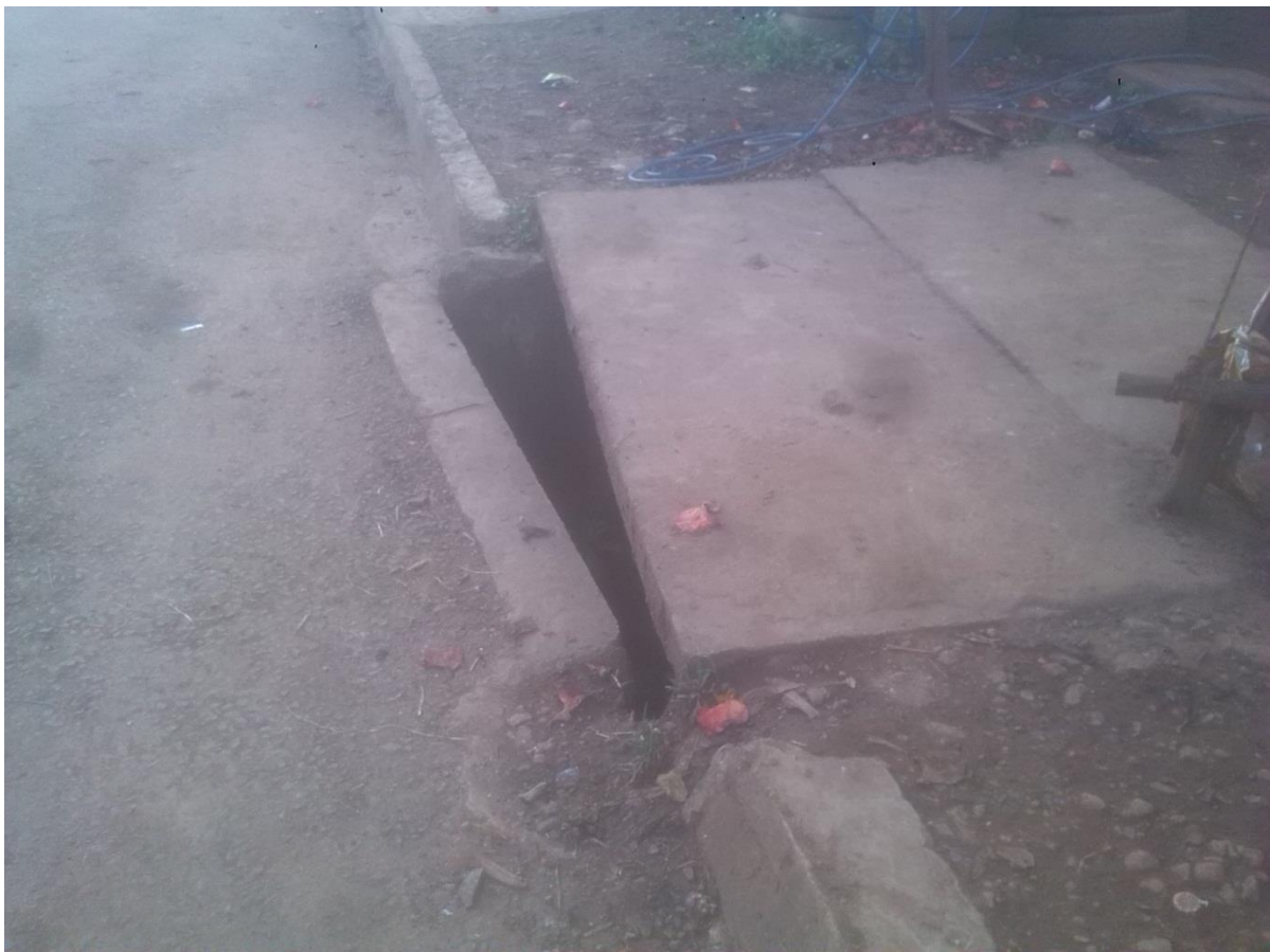
Figure 13 Drainage inlet structure construction problems and manhole cover not fit
