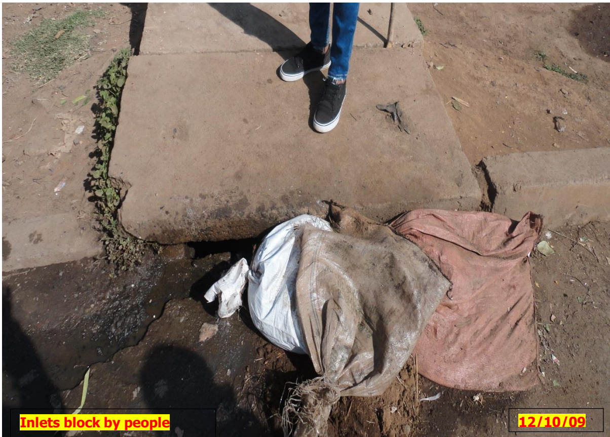
Figure 4.22 Waste water inter to manhole inlets across on pavement structure
