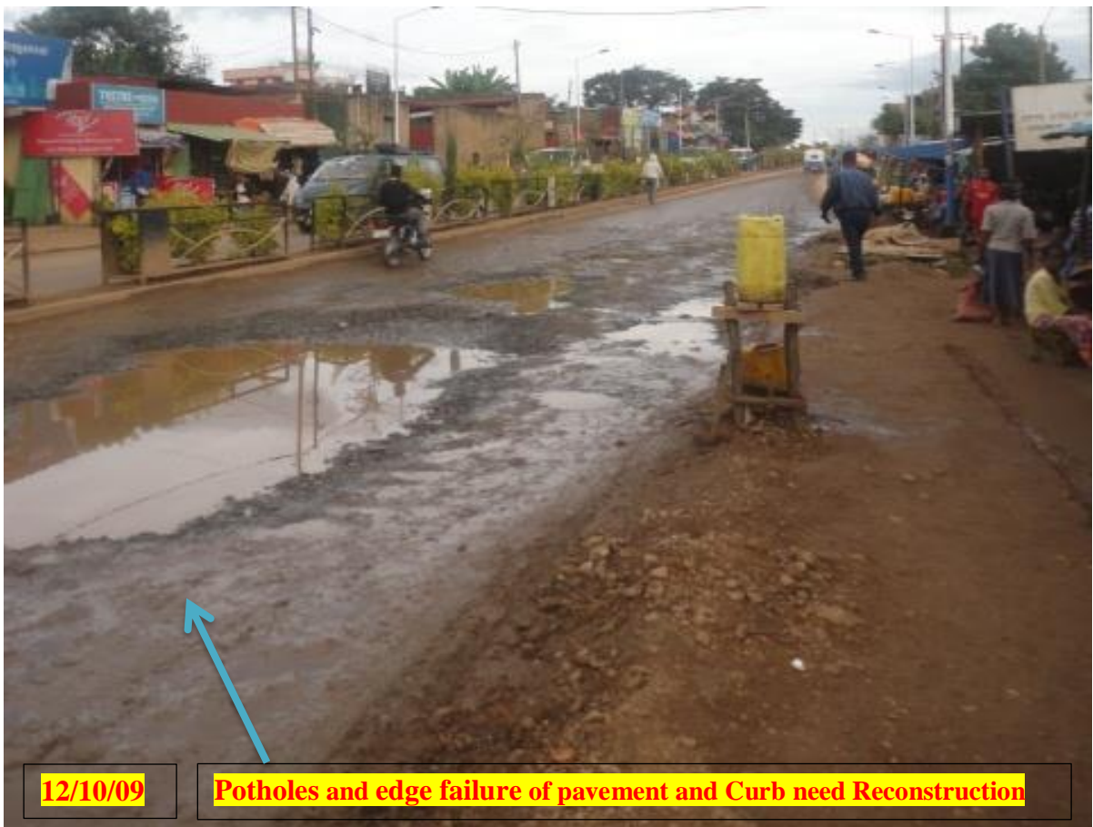
Figure 4.21 shows that pavement failure and inlets doesn't work (in front of genu hotel)
