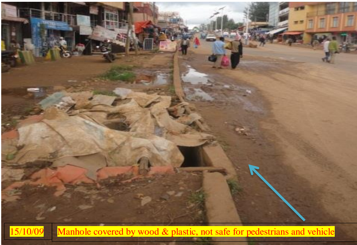
Figure 4.6 shows inlets closed by debris and connected with toilets, around genu hotel
