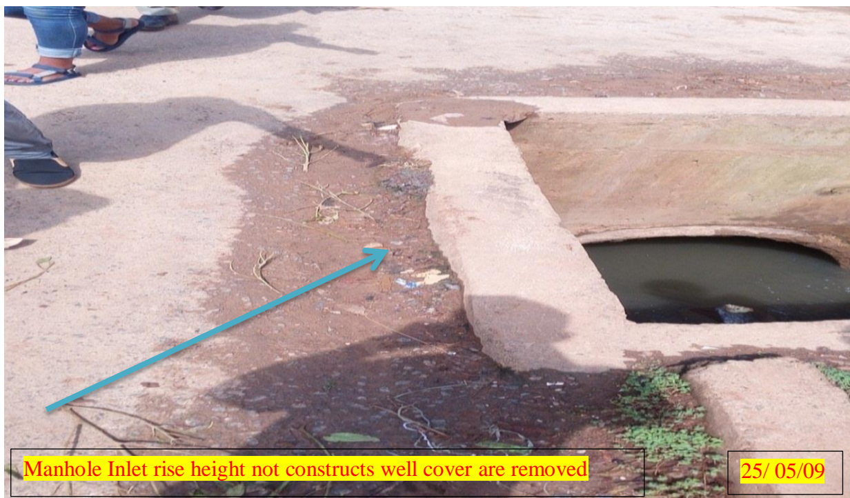
Figure 4.11 inlets contract over design and manhole cover (around feidi roundabout)
