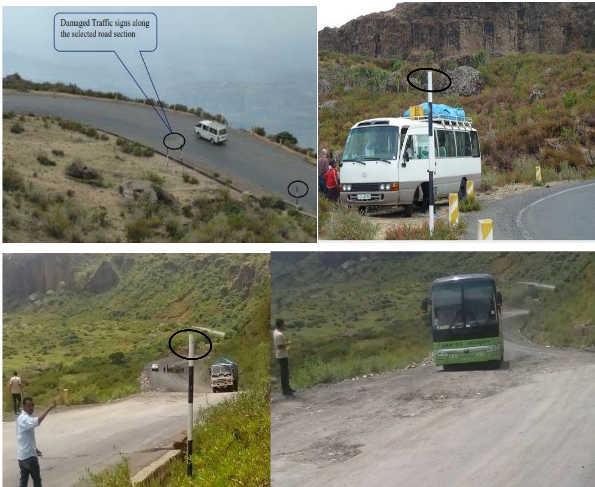
Figure 3.12: Field photos with damaged traffic signs and wornout pavement surface.
