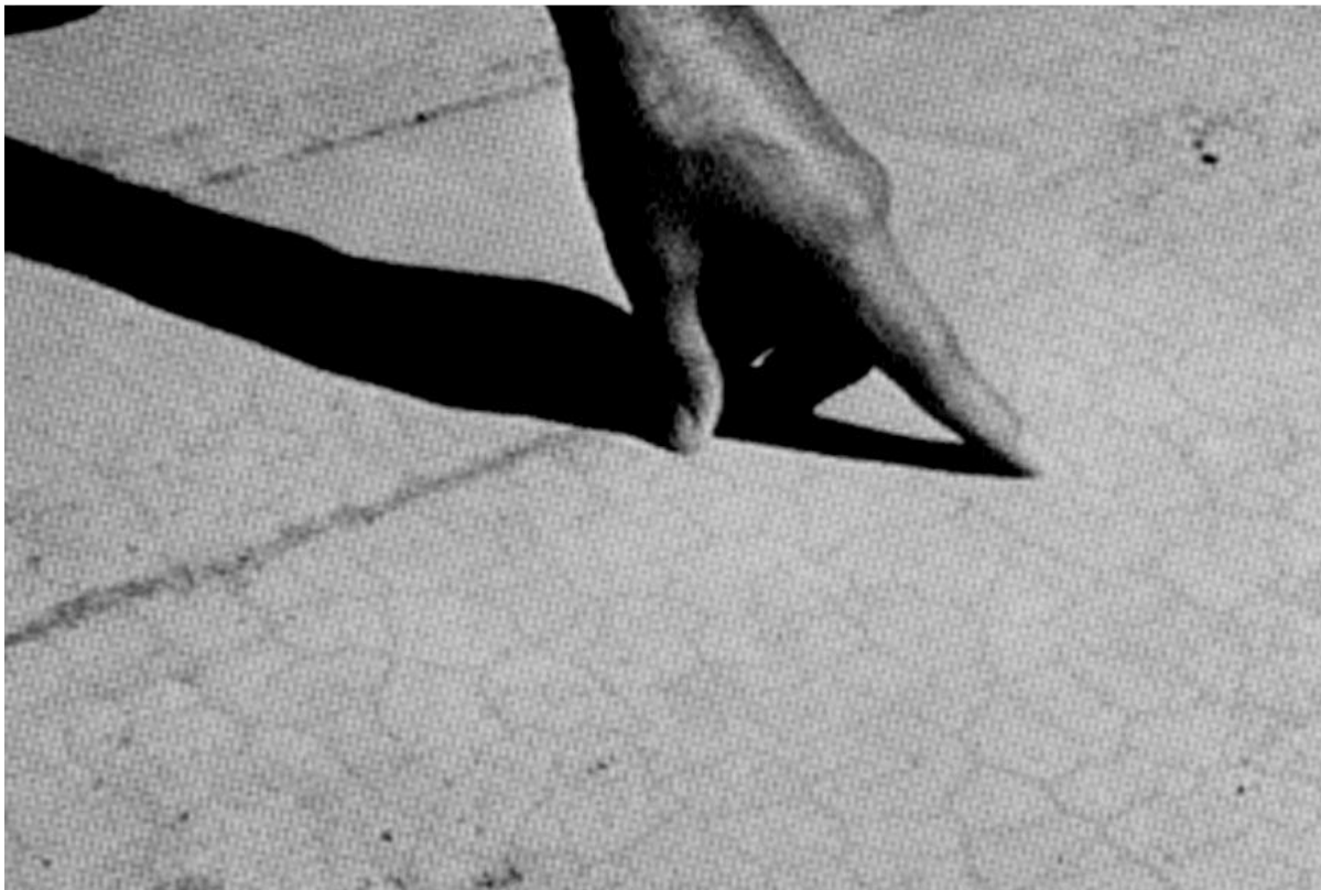
Figure 3 Crazing, a network of fine surface cracks.
