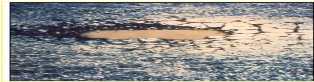
Figure 2.11:- Potholes (Catalogue of Road Defects (CORD) January 2013).
