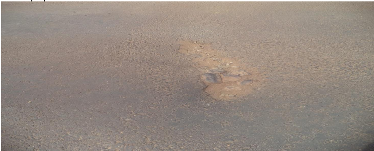
Less sever potholes
