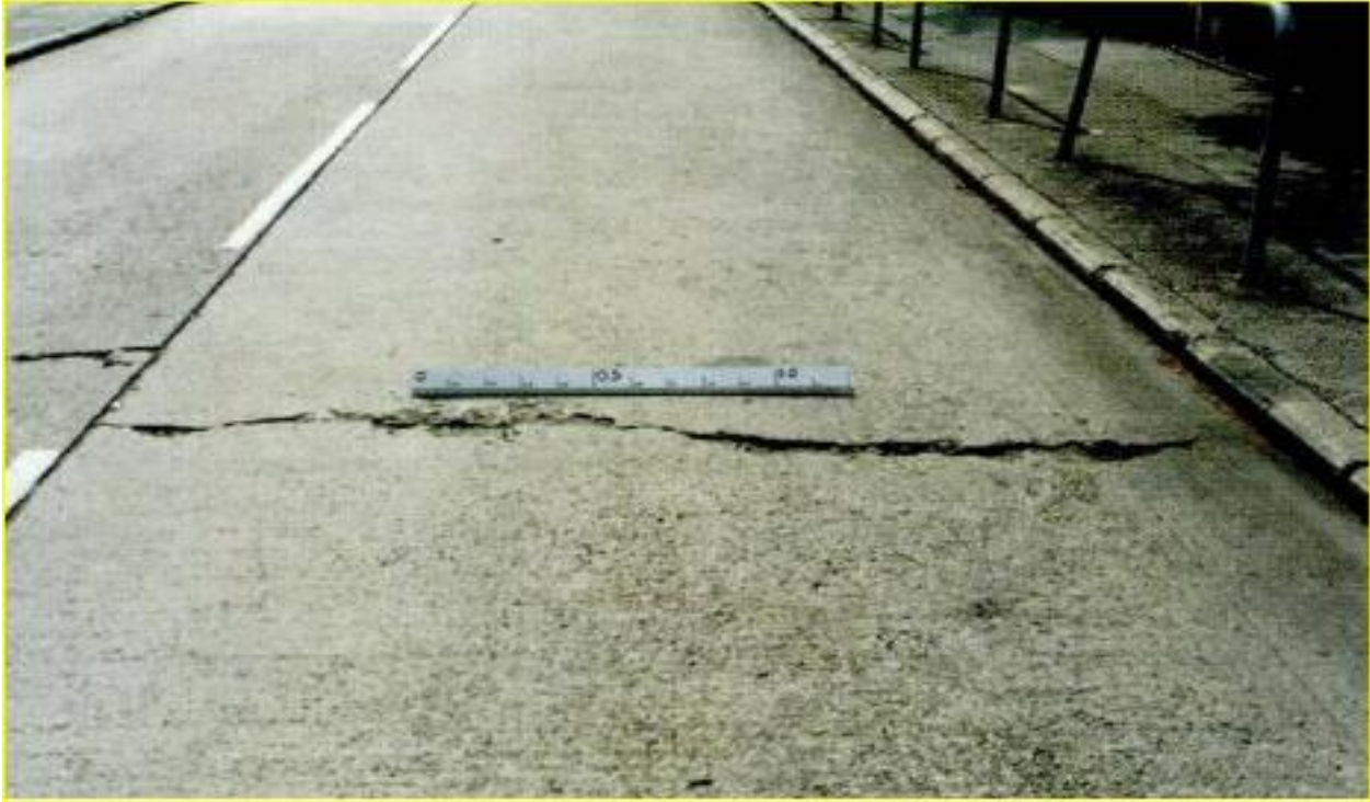
Figure 2.3. Transverse cracks (Catalogue of Road Defects (CORD) January 2013).
