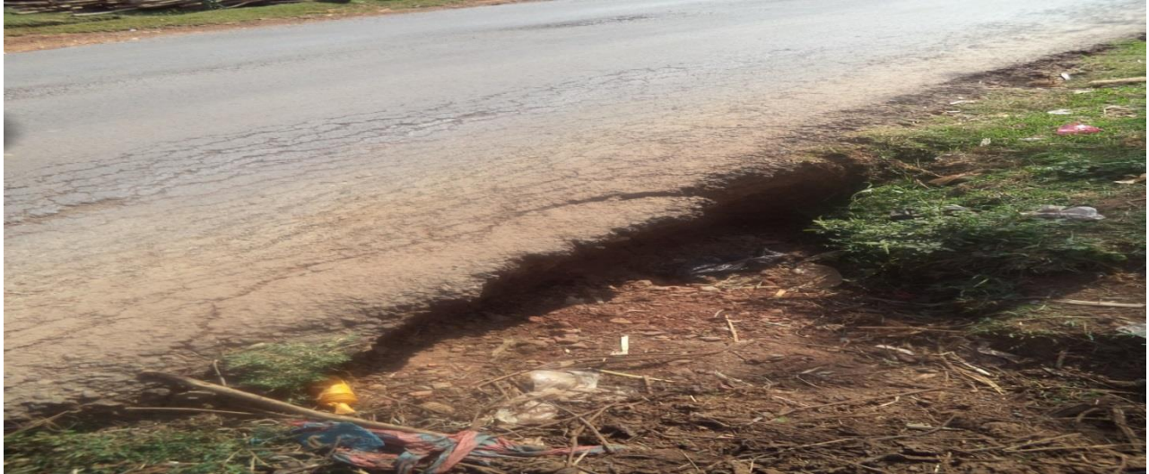
Absence of shoulder support and drainage problem
