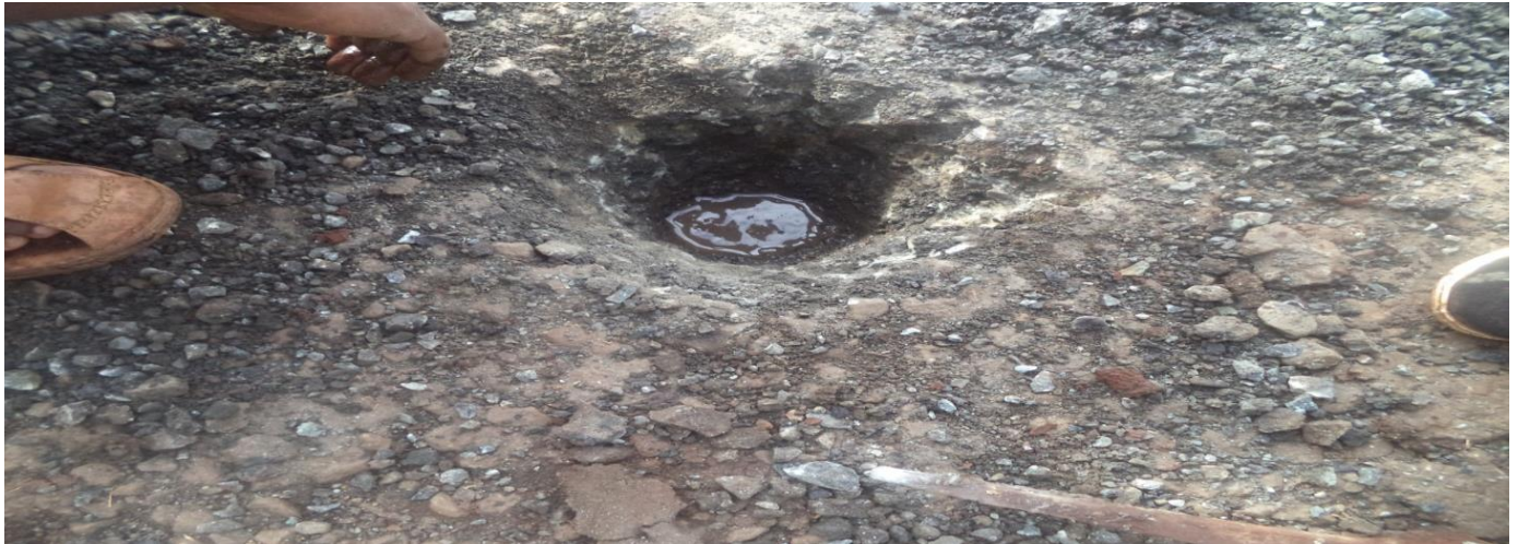
Moisture condition on pavement layer
