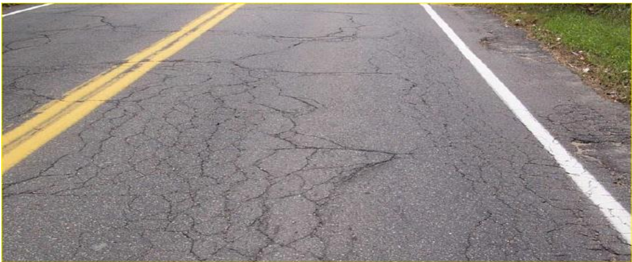
Figure 2.1: Alligator cracks (Pavement Distress Identification Manual, July 2011)
