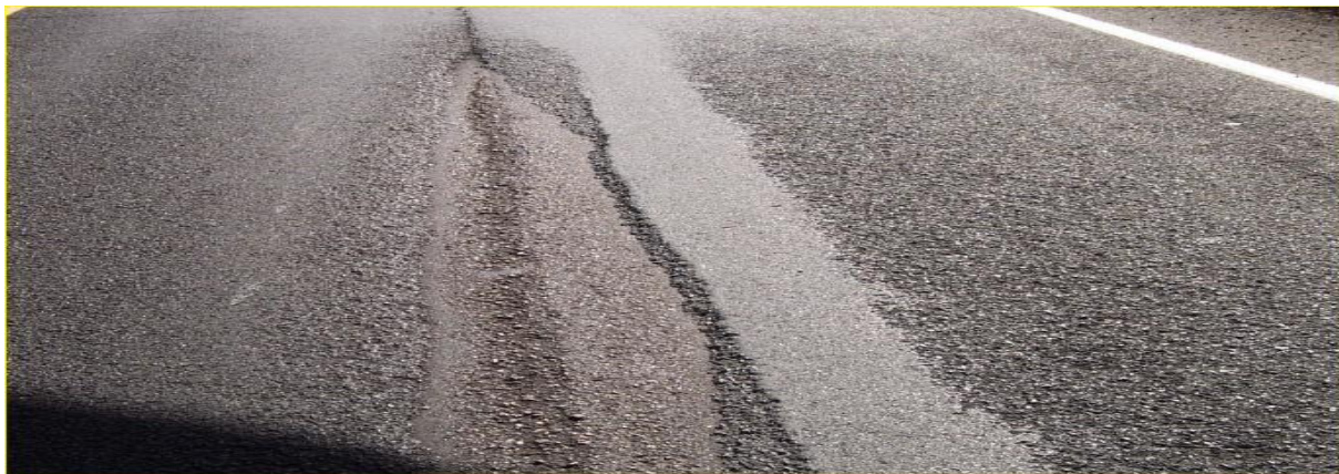
Figure: 2.13 Ravelling (Catalogue of Road Defects (CORD) January 2013).
