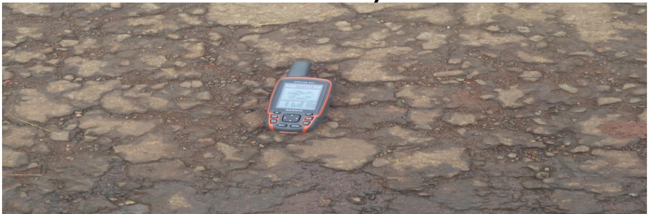
Locating of Defects using GPS
