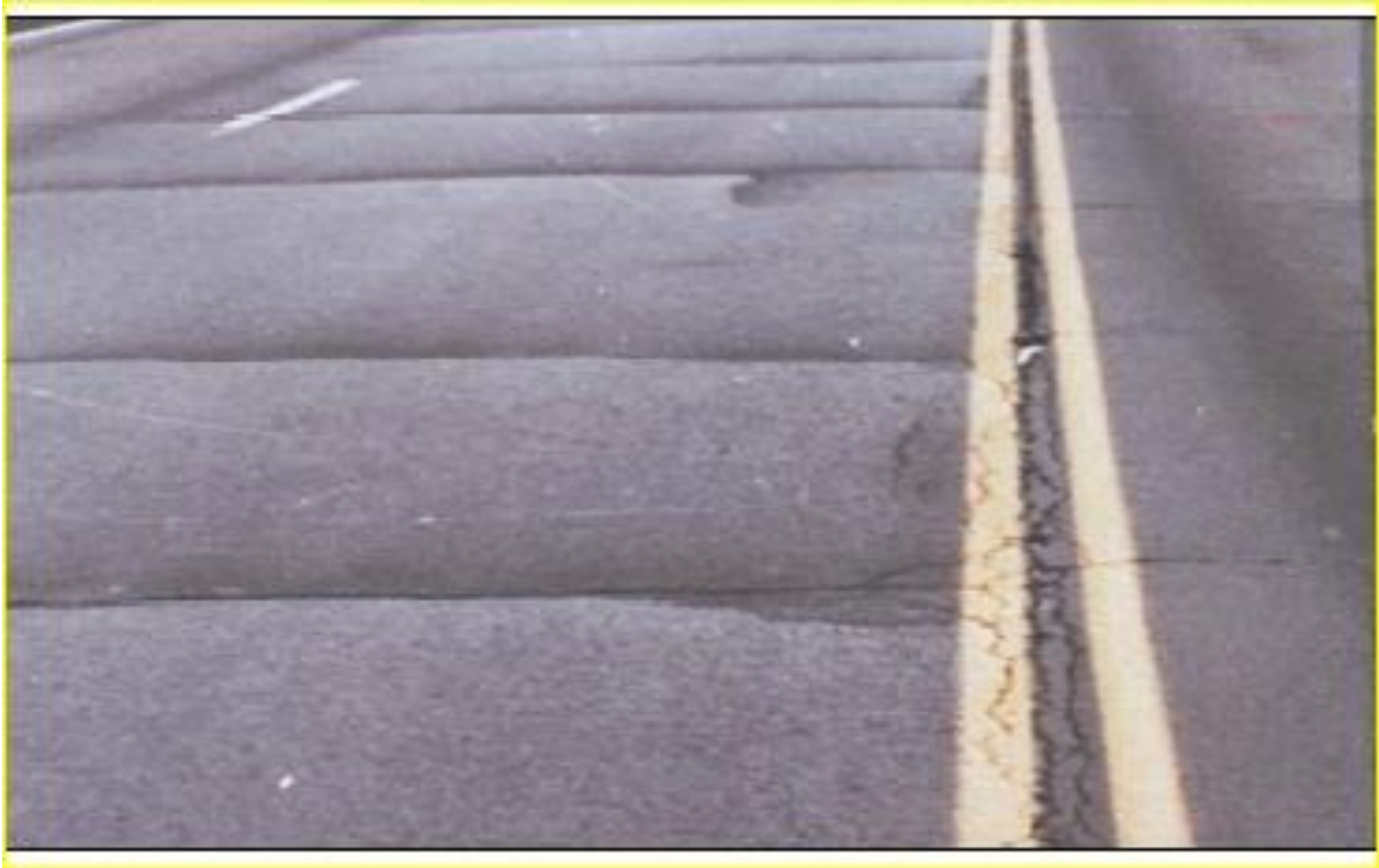
Figure 2.6. Reflective cracking (Pavement Distress Identification Manual, July)
