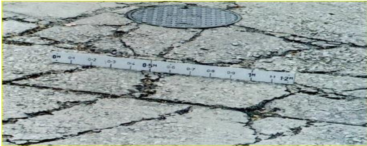
Figure 2.4. Block cracks (Catalogue of Road Defects (CORD) January 2013).
