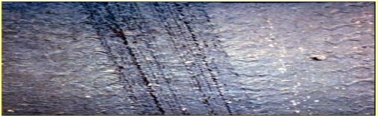
Figure:2.14 Bleeding(Catalogue of Road Defects (CORD) January 2013).
