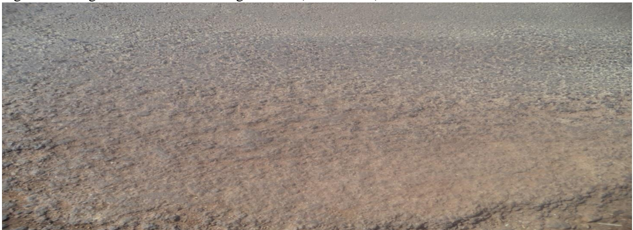
Figure 4.5 longitudinal cracks and edge cracks (29-Nov-15)
