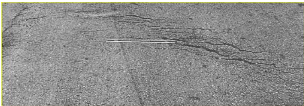
Figure 2.5. Slippage cracks (Catalogue of Road Defects (CORD) Division January 2013).
