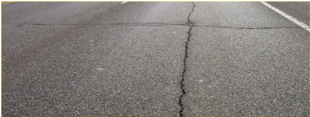
Figure 2.2. Longitudinal cracks (Pavement Distress Identification Manual, July 2011).
