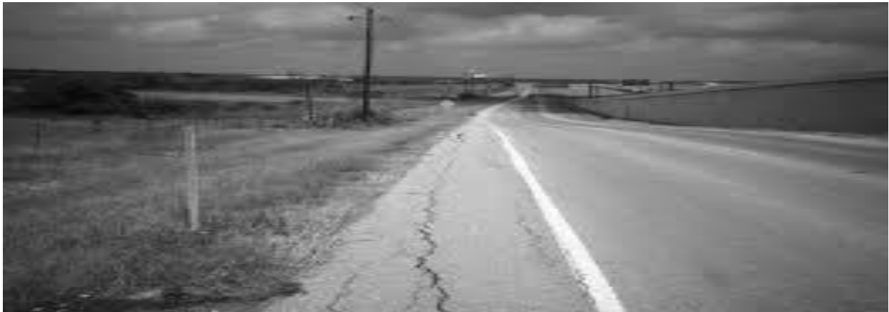
Figure 2.7. Edge cracks (Pavement Distress Identification Manual, July 2011)
