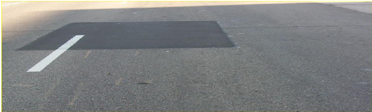
Figure: 2.12 patch(Catalogue of Road Defects (CORD) January 2013).
