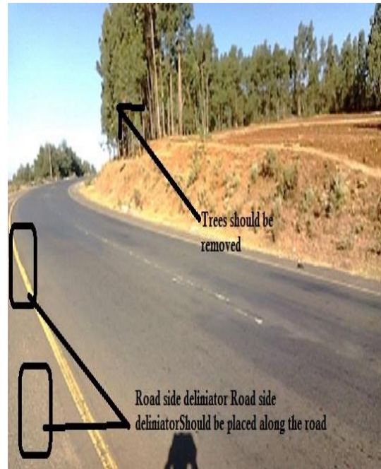
Figure 4.14 Menagesha (22km) after counter measure is applied
