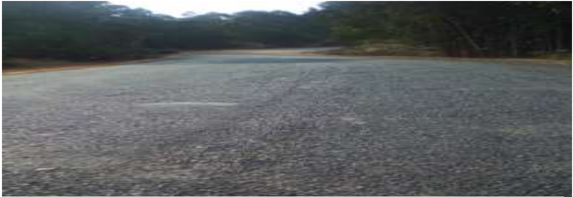
Raveling of asphalt surface
