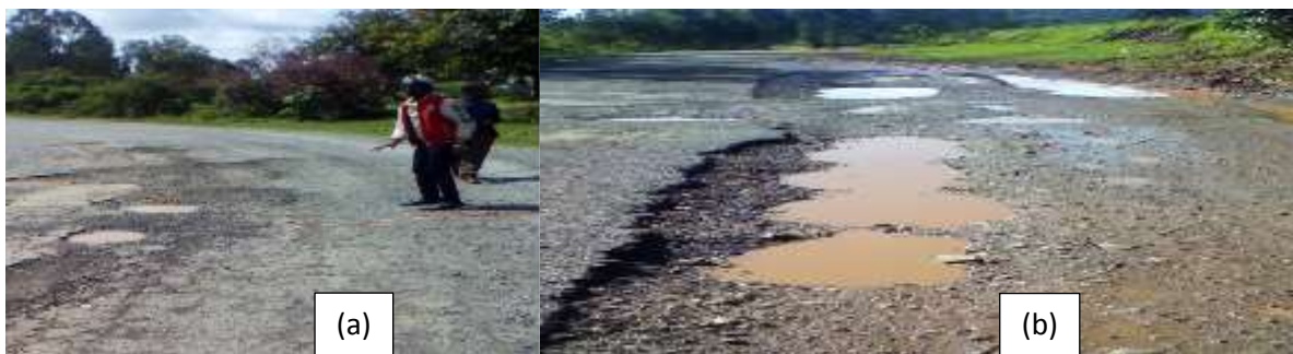
Figure 4.3 Potholes (a) and Corrugation (b)
