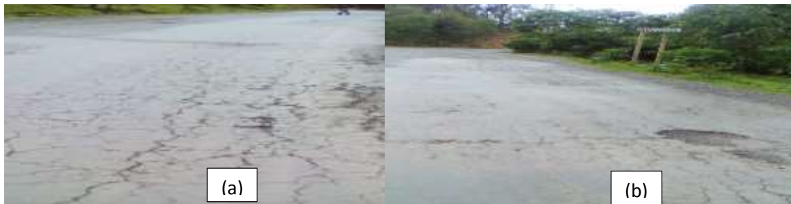
Figure 4.5 Alligator Crack (a) and (b)
