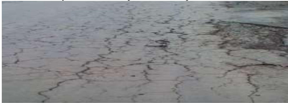
Figure 2.2: Alligator cracking, [From study Area].
