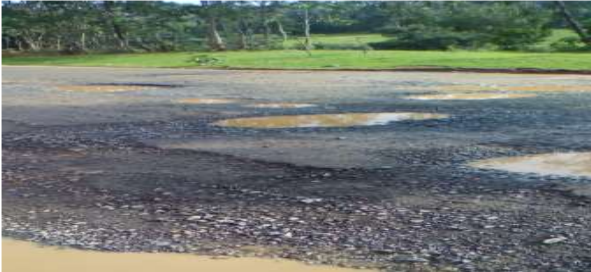
Disintegrations and Potholes
