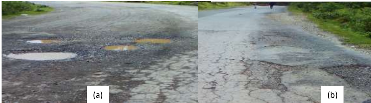
Figure 4.1: Pothole (a) and Patching (b)
