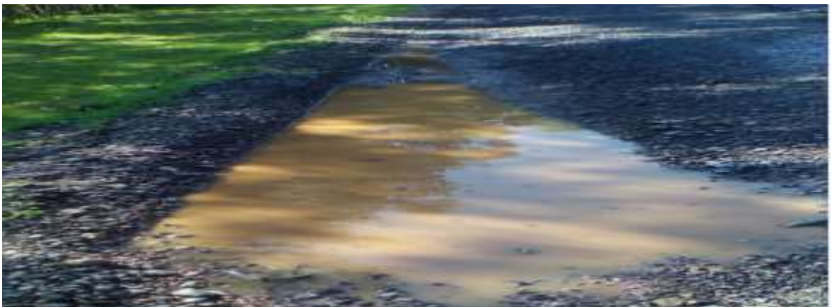
Rutting on side
