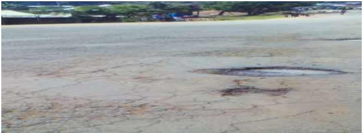
Potholes and Alligator crack
