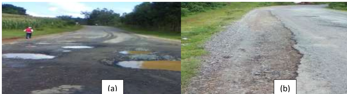
Figure 4.6 Potholes (a) and Edge failure (b)
