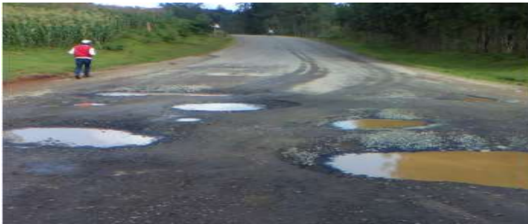
Figure 2.11 Potholes, [From study site].
