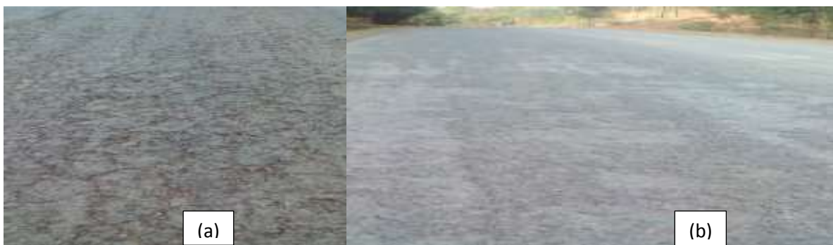
Figure 4.2: Raveling (a) and stripping (b)
