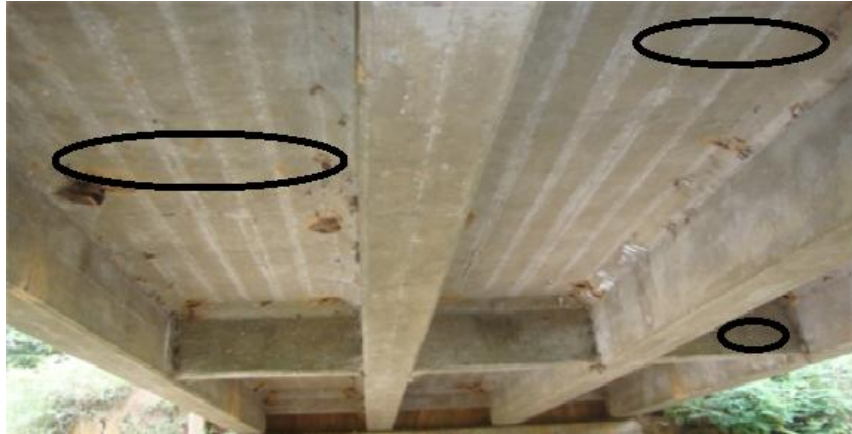
Figure 4.6: Marked delaminated areas of Sheta River Bridge deck
