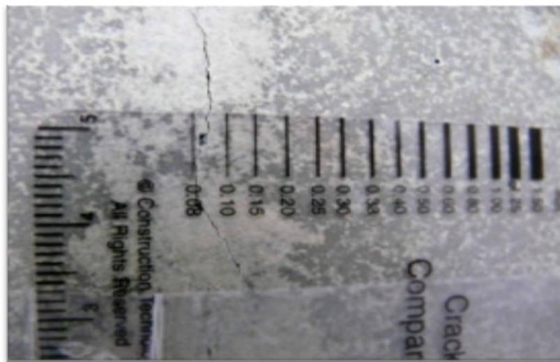
Figure 2.5: Typical crack width measurement on bridge deck [12]
