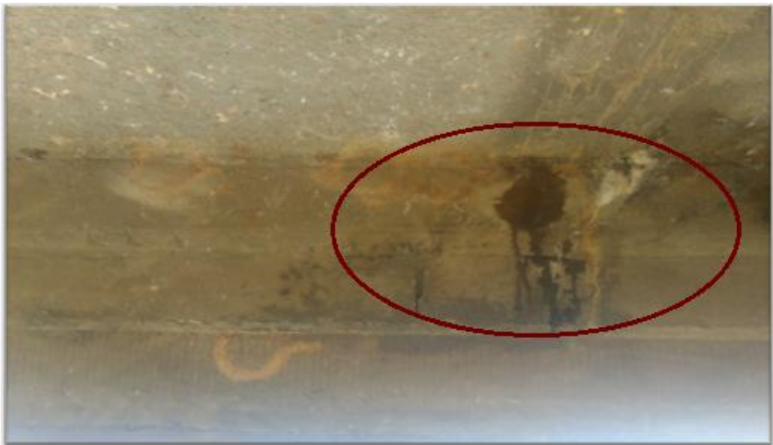
Figure 4.2: Visible leakage at cracks underneath of deck slab
