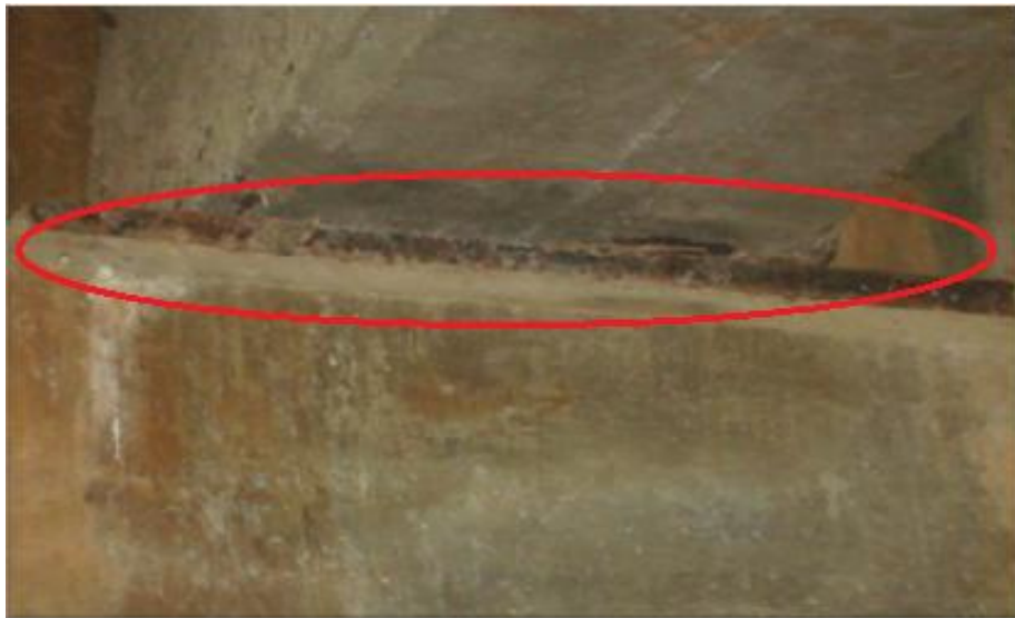
Figure 4.13: Corrosion of steel plate bearing
