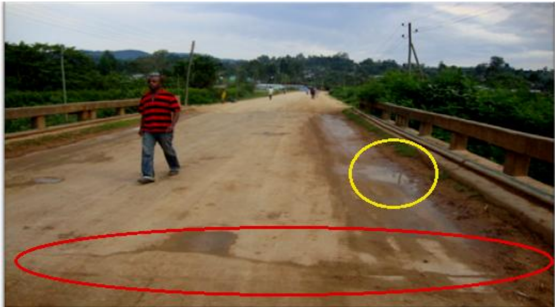
Figure 4.1: Visible transverse bridge deck cracking and deposited silt
