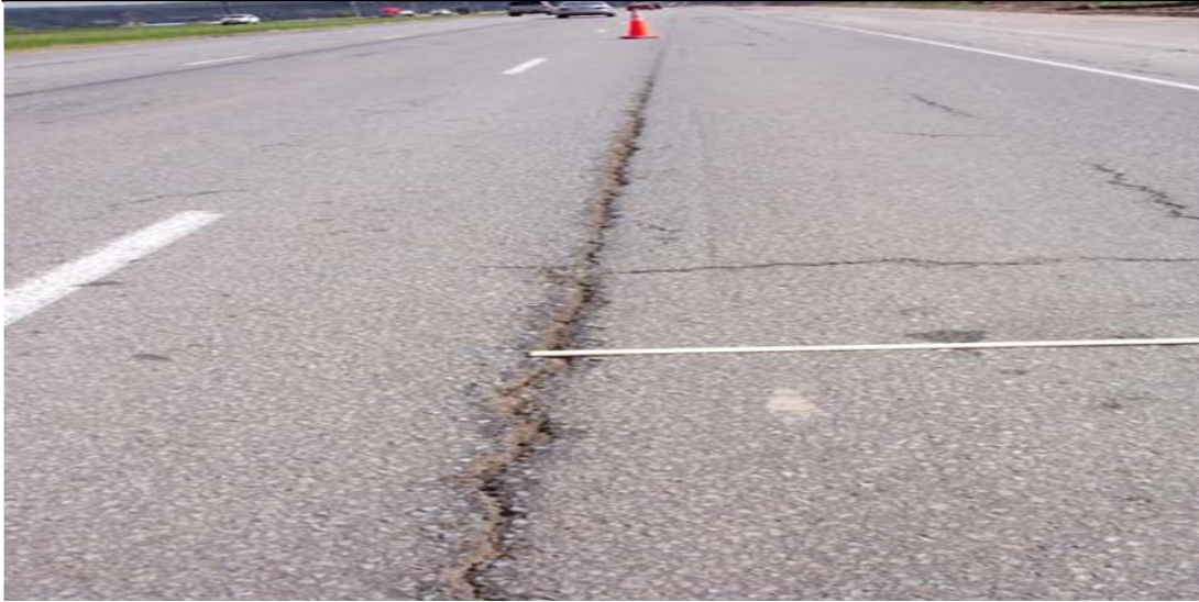
Fig. 2.4: High severity Longitudinal Cracking
