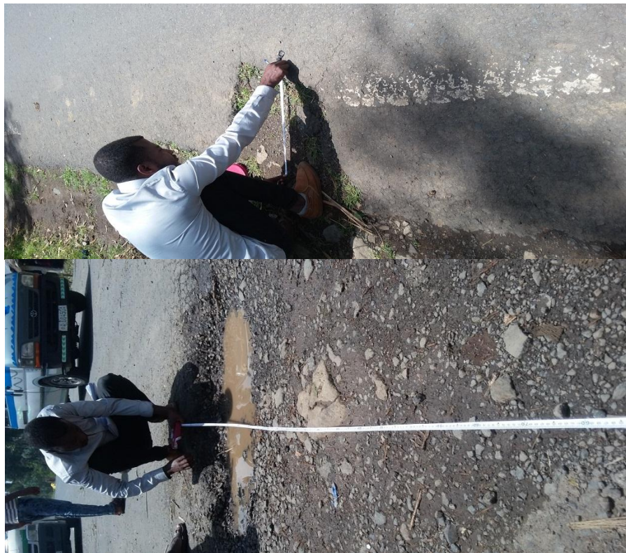
Fig. 3.3 Edge cracking measurement
