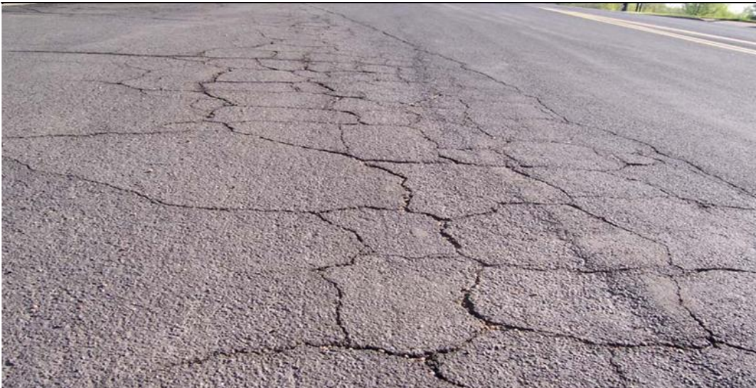
Fig.2.3: High severity alligator cracking
