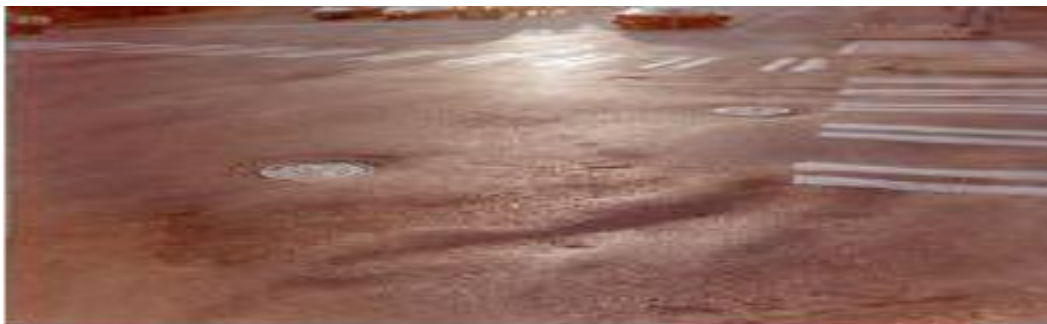
Fig.2.8: High severity Corrugation
