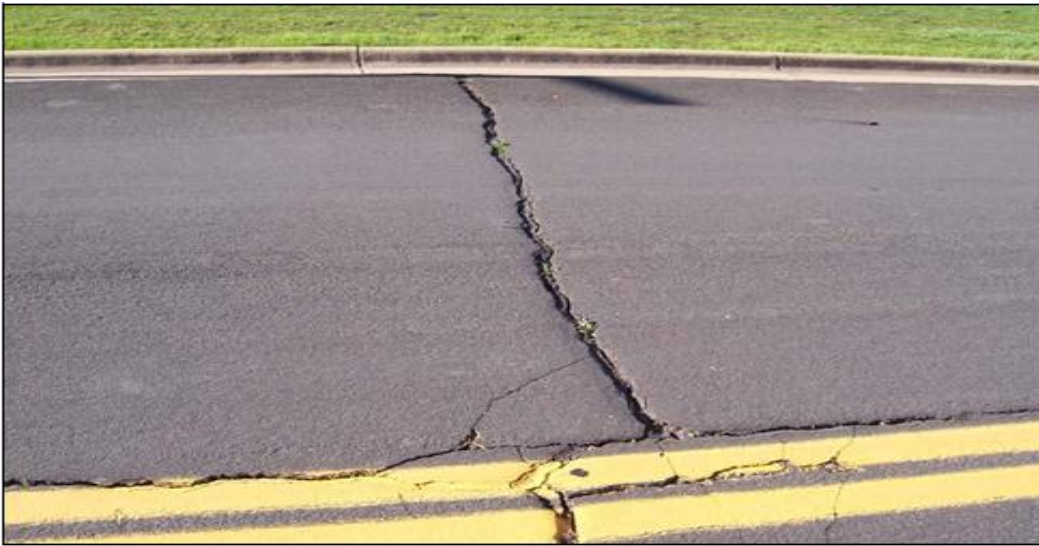
Fig. 2.5:High severity Transverse Cracking
