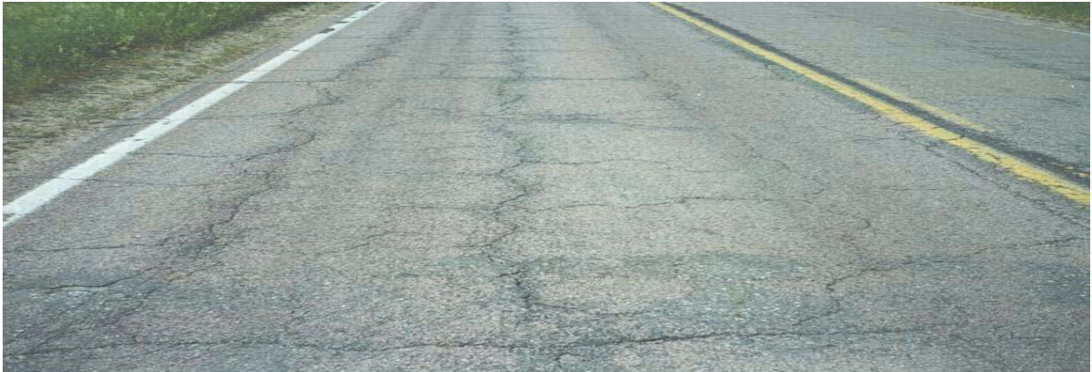
Fig. 2.9: High severity block cracking
