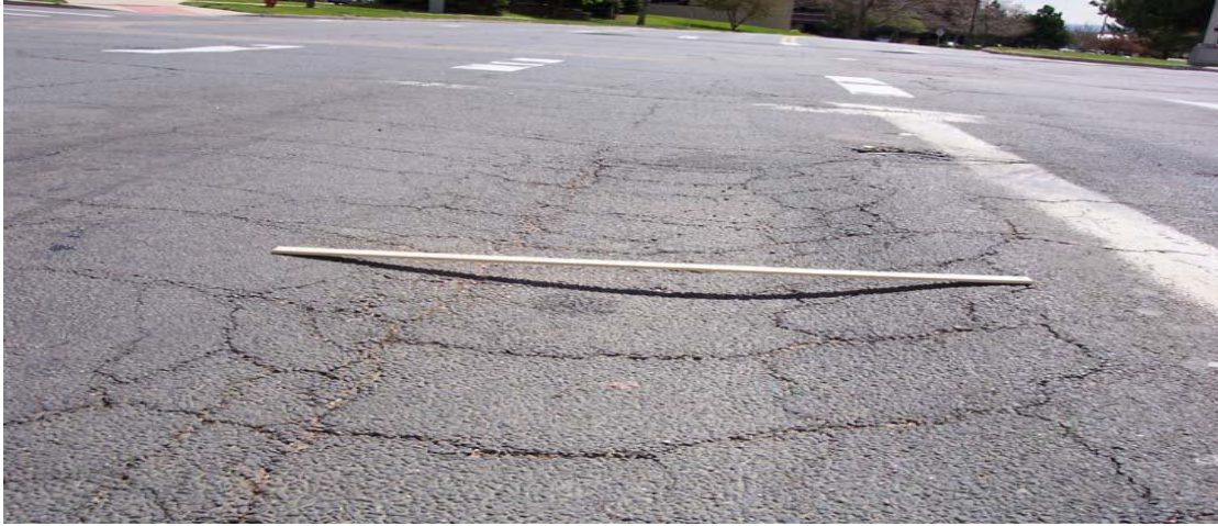
Fig.2.2: High severity rutting
