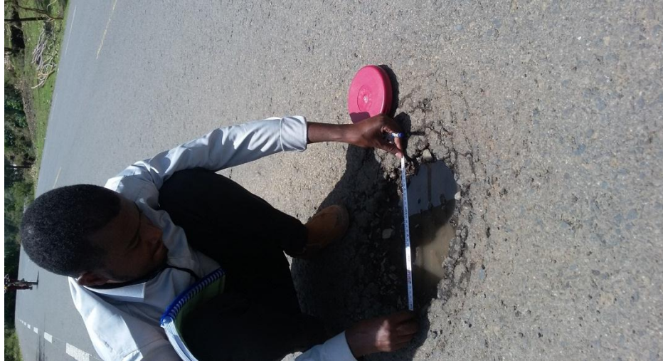
Fig. 3.4 Potholes counting and measurement
