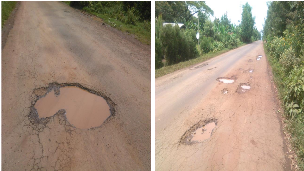
Fig.2.1. Potholes (Location around Bulbulu Station 40+100)
