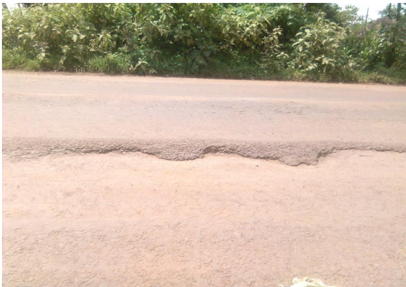
Fig.2.4. Corrugation (Location Bulbulo station 39+240)
