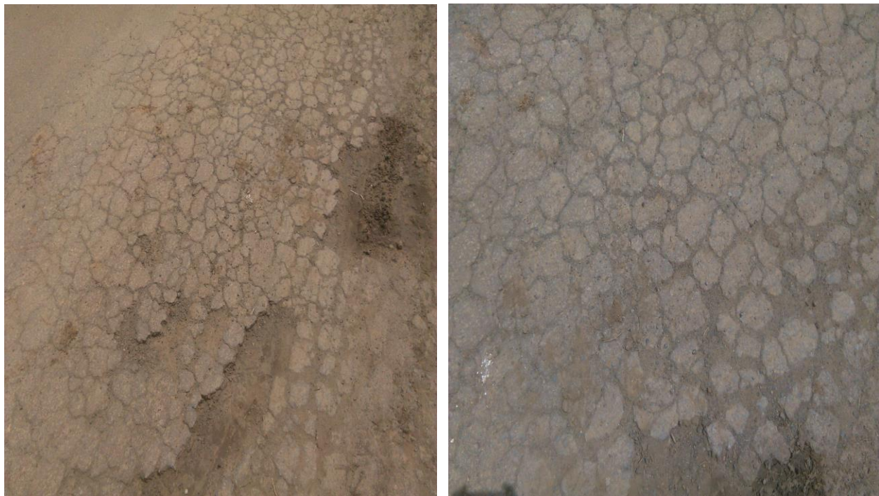
Fig.2.2. Alligator or Fatigue cracking (Location Gembe station 33+420)
