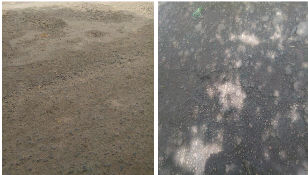
Fig.2.6. Raveling surface (Location- Dabesa & Harro- station 26+650 &29+450)
