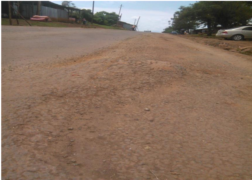
Fig.2.3. Shoving (Location Gembe-station 33+050)
