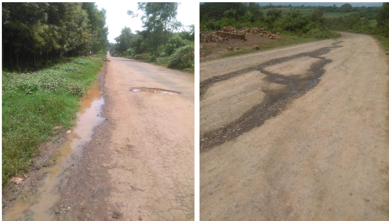
Fig.2.5. Poor drainage effect on the road surface (Location Bulbulo & Gembe)
