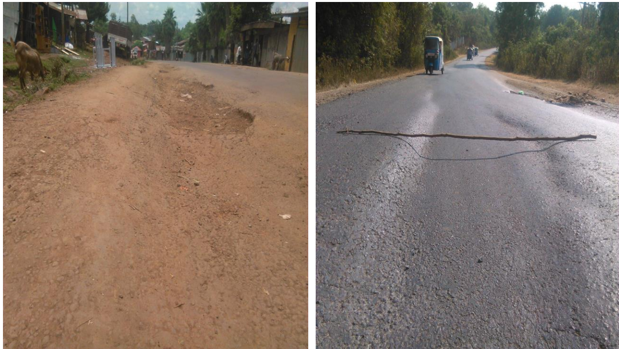
Fig.2.7. Rutting (Location - Gembe & Agaro)
