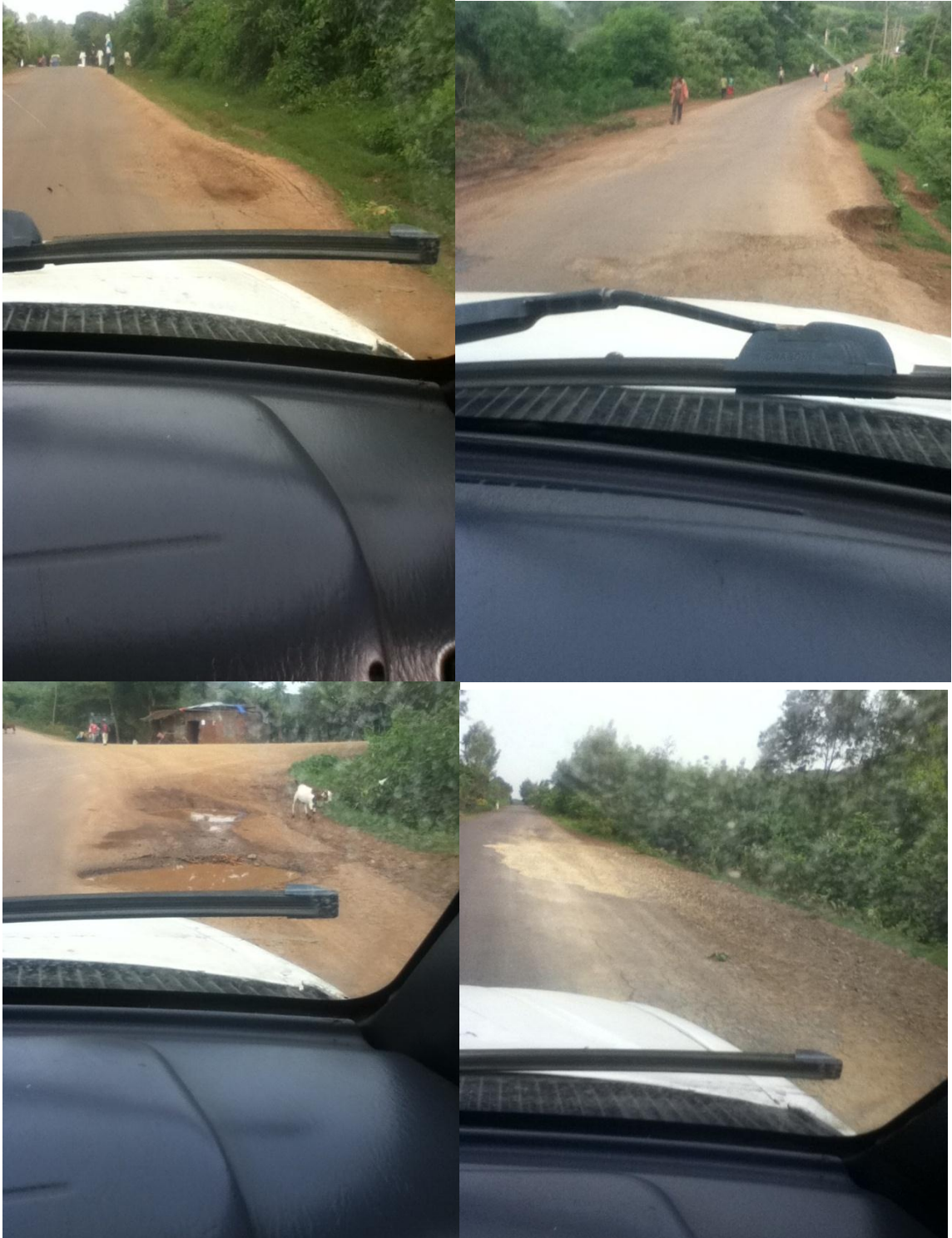
Drainage and vegetation problems
