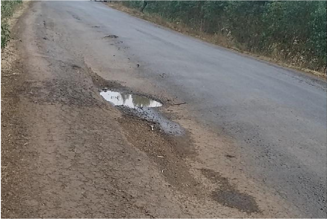
Potholes, settlement and cracks at 62+900
