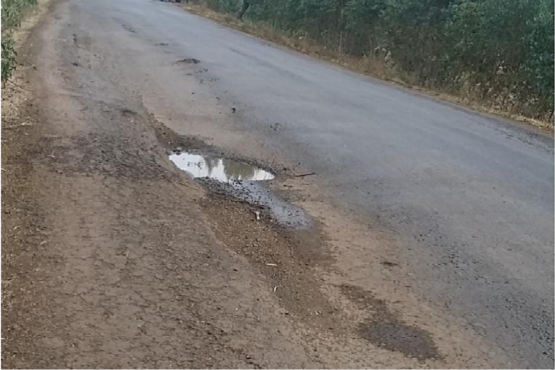
Potholes, settlement and cracks at 62+900
