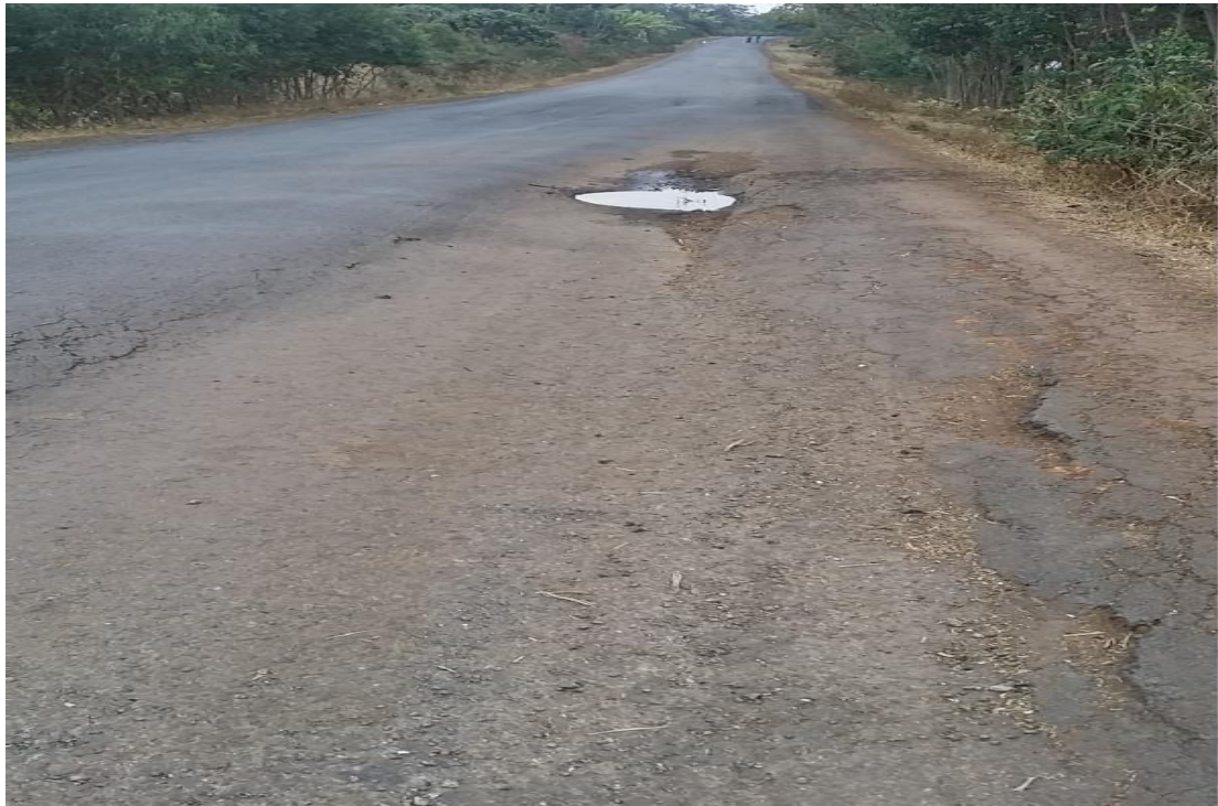
Pothole cracks and Sag in asphalt at 62+300
