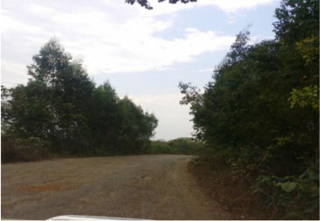
Disintegration, Raveling, loss of pavement material along the pavement at station 65+000
