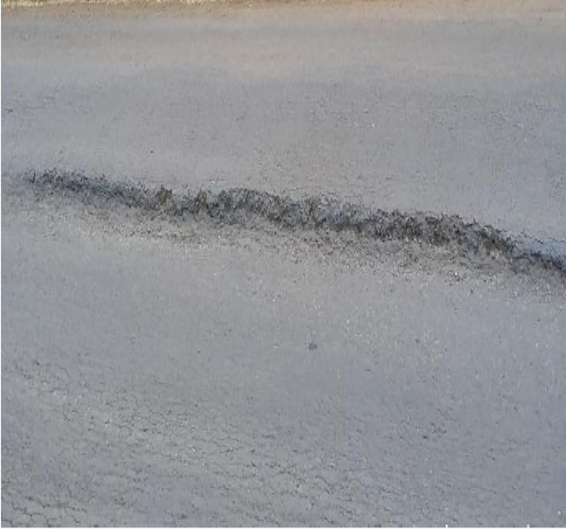
Cracks and settlement at 62+600
