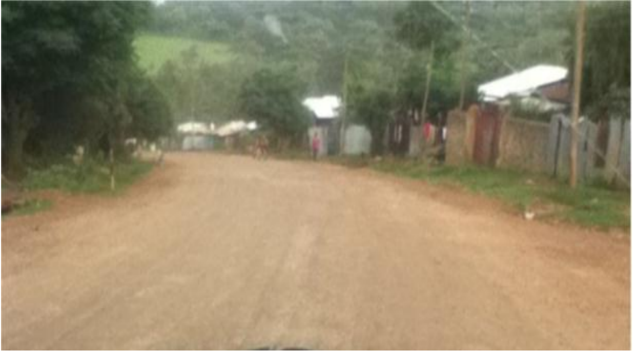
Disintegration of road at station 65+300
