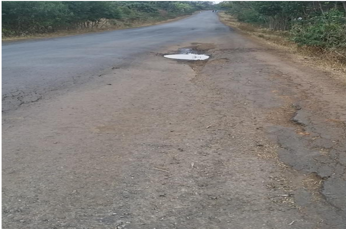
Pothole cracks and Sag in asphalt at 62+300
