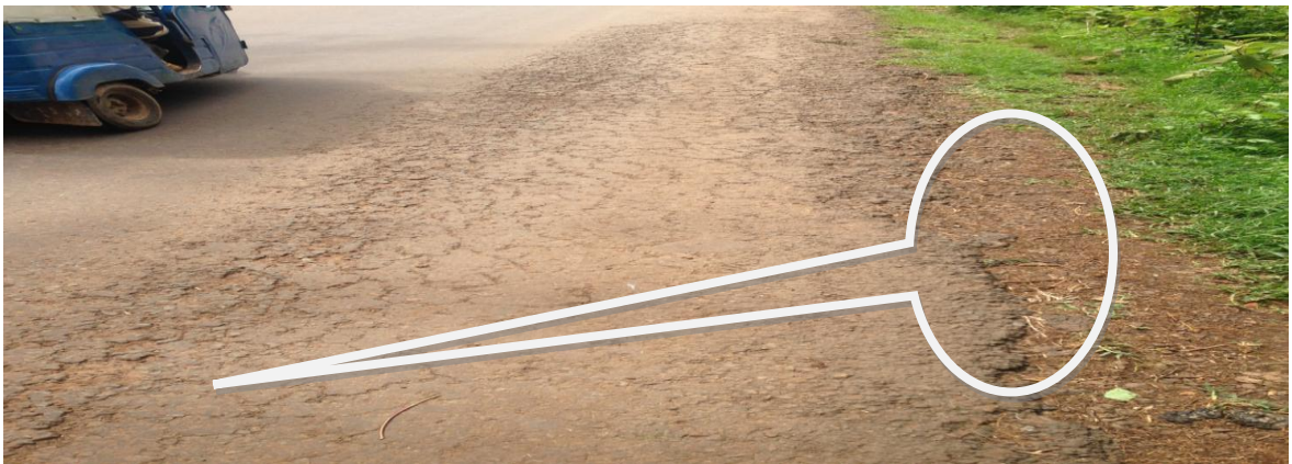
Figure 4 1: Alligator Crack at the edge
