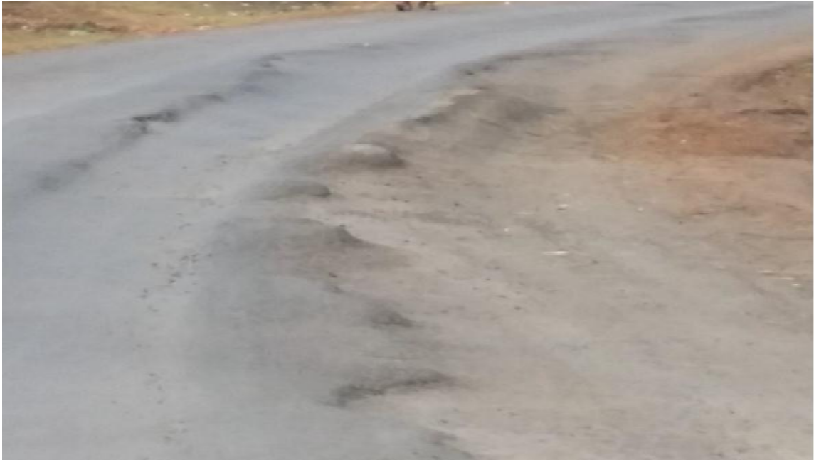
Figure 4. 6: longitudinal deformations, settlements and Rutting in asphalt pavements at 65+000.
