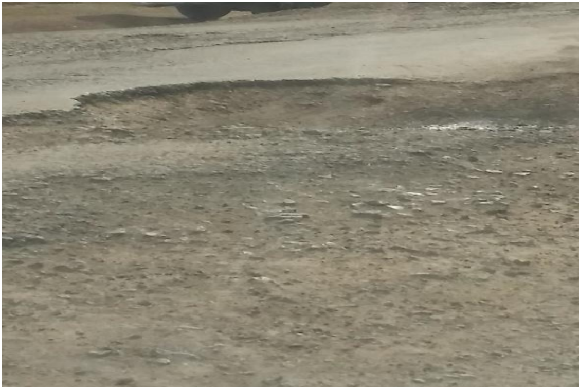
Figure 4 5: Exposed base material of road at station 44+200
