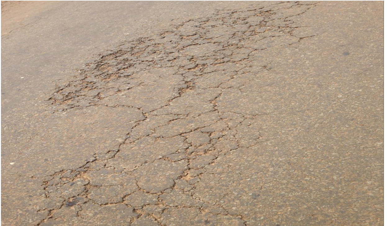
Figure 4 2: Alligator Crack at the center
