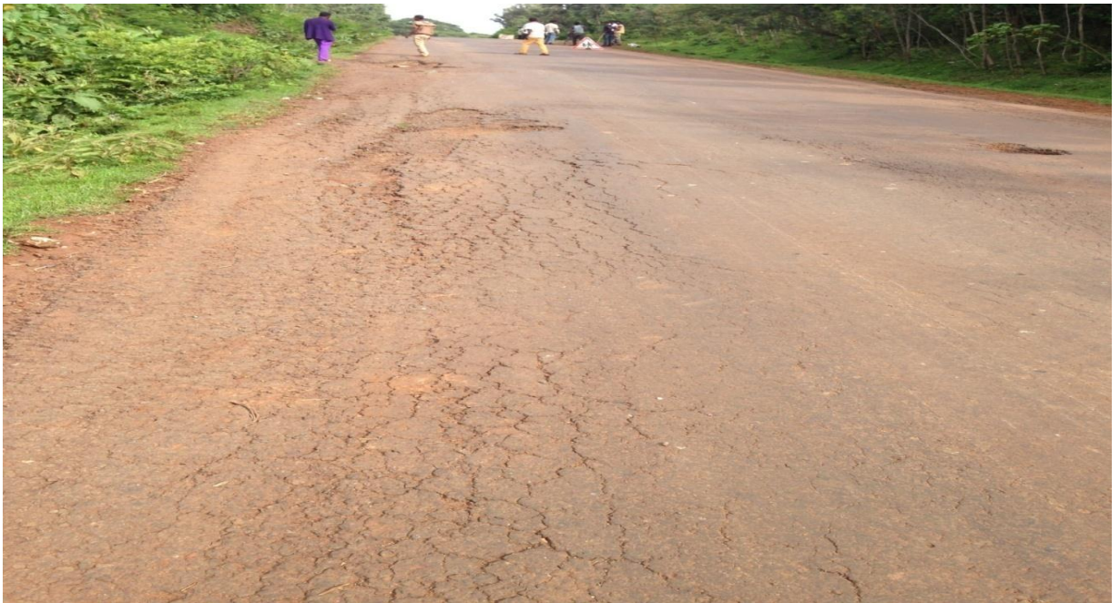
Figure 4 3: Crack, Potholes, vegetation cover at side walk and shoulder
