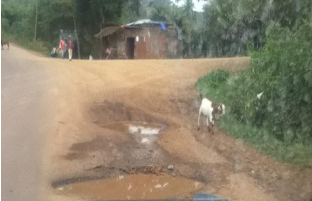
Figure 4 4: Potholes at the edge of the road
