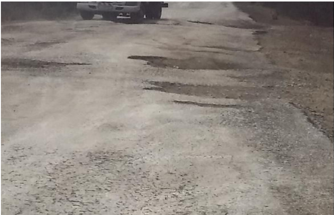
Crack, Potholes and loss of pavement material along the pavement at 43+600.
