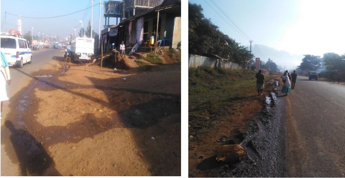
Figure 3. 7 : Field photo with absence of drainage structure at str 1 & 2.
