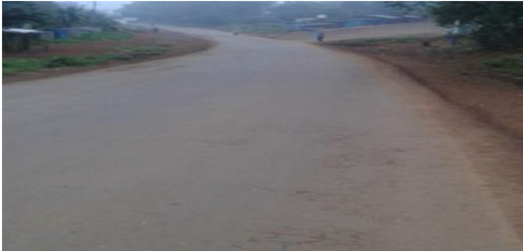
Figure 3. 8:Field photo with improper junction & missing of traffic sign & stretch 2
