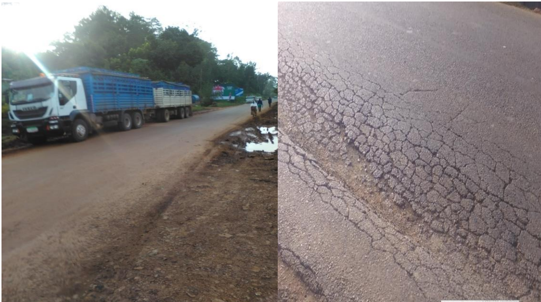
Figure 3. 10 : Field photo with absence of parking area & pavement distress
