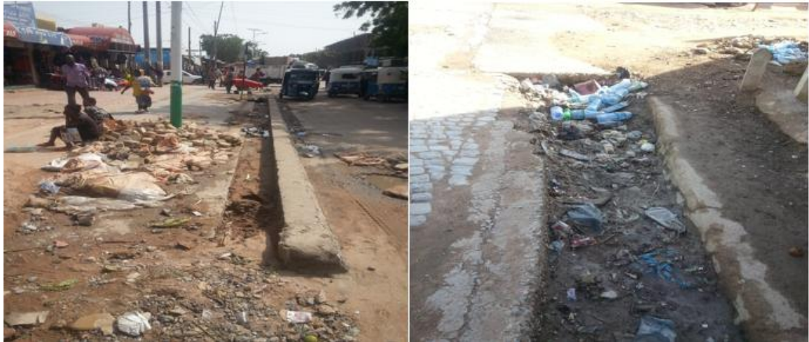
Figure 4.4: Poor roadside drainage in the study area
