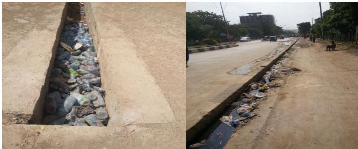
Figure 4.11:Filled roadside due to illegal waste disposal
