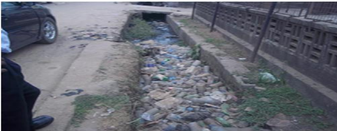
Figure 2.1:Blocked drains because of abuse of drains with waste deposits
