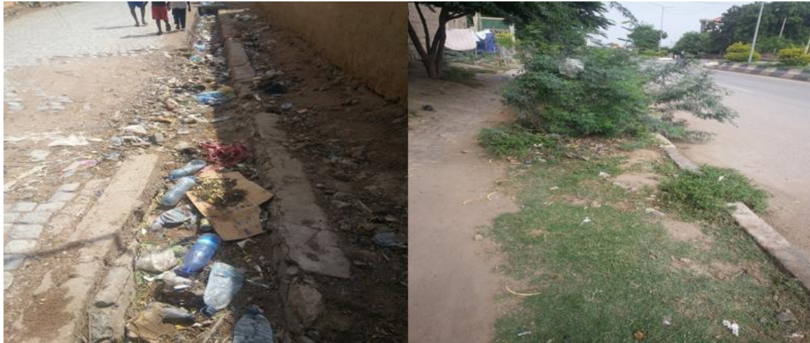
Figure 4.13:Blocked roadside drain due to waste and filled with grasses and sediment
