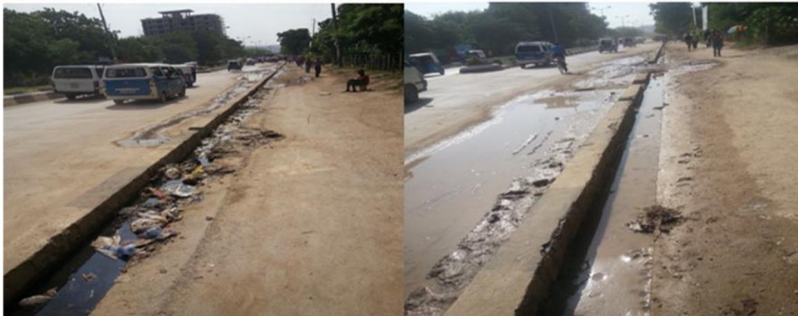
Figure 3.2:Blocked roadside drainage due to waste disposal and sediment accumulation
