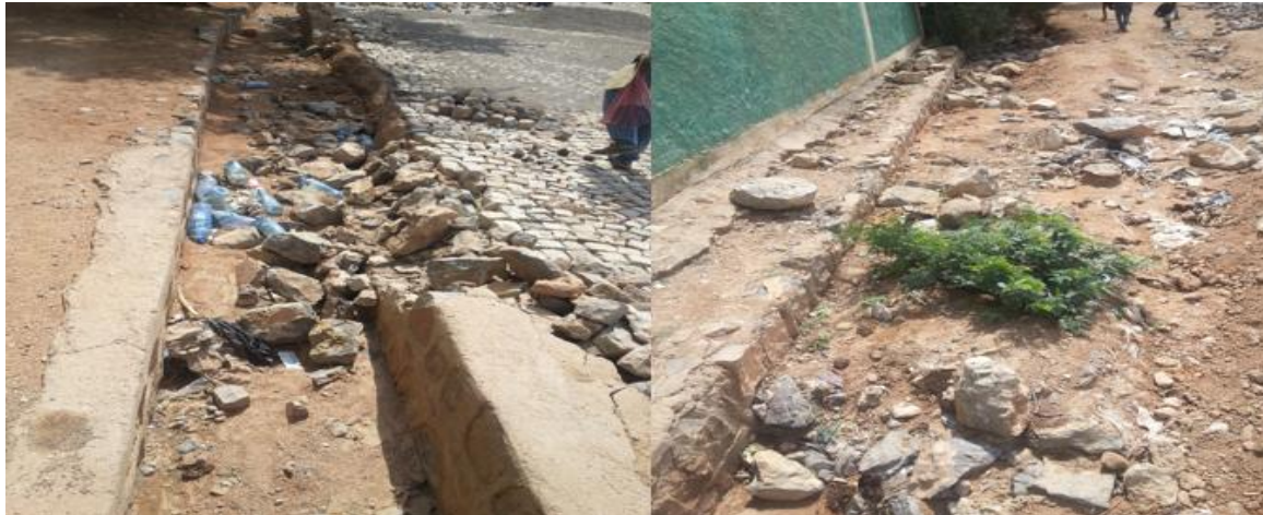
Figure 4.15: Damaged roadside drainage due to cobble stone construction
