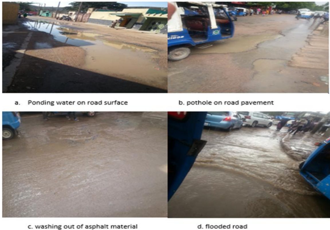
Figure 4.16: Existing condition of road pavement in study area
