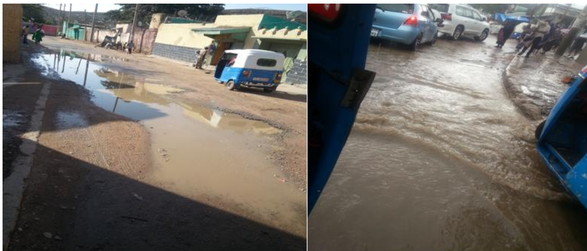
Figure 4.9: Ponding of water on carriageway and the overflow of run water
