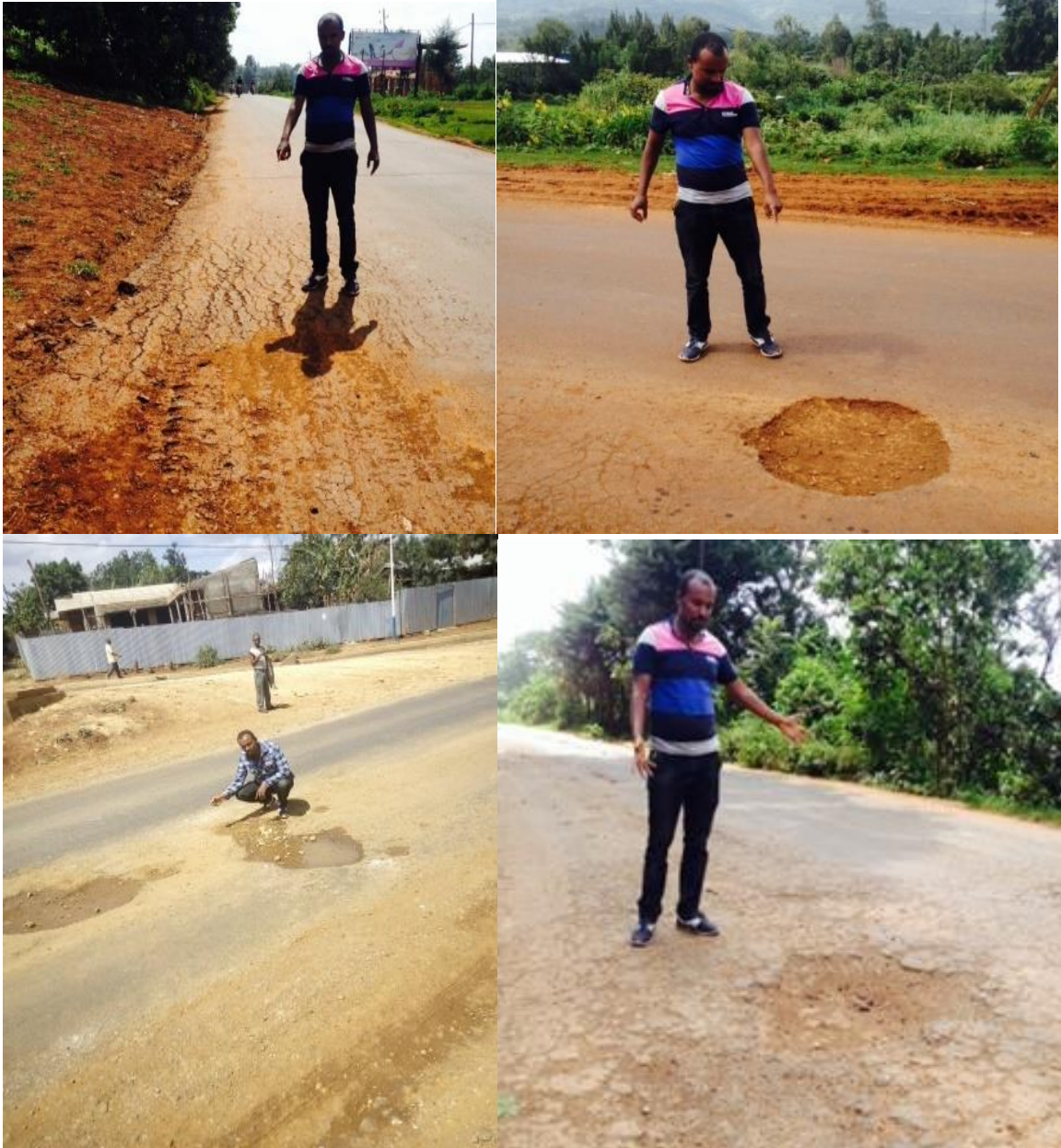
Figure 1.1 Photos for the current existing condition of the studied stretch pavement (photo captured date 08-04-2017 @2:00 – 5:00p.m.)
