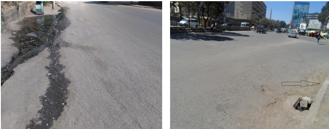
Fig. 1.5: Photo, Repeated overlay construction making asphalt overall thickness higher than the curbstones and creating drainage problems in front of the Ambassador Hotel.
