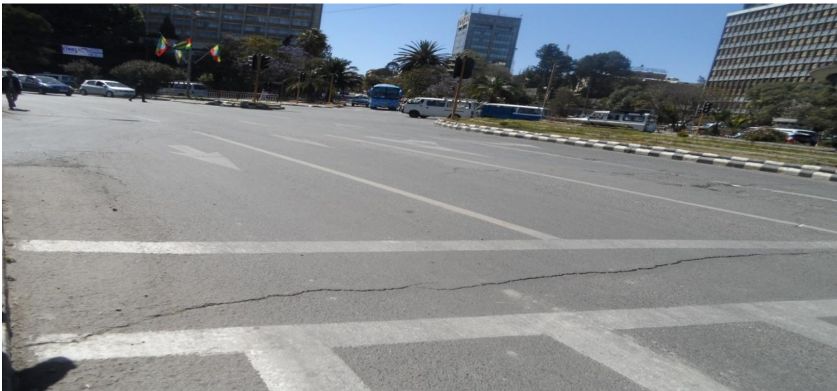
Fig. 4.1 Photo: Major Crack at the National theatre 1 site (before application of the overlay)
