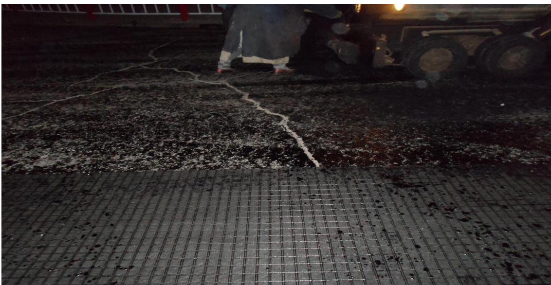
Fig.3.6: Photo: Image showing an untreated major crack running through both the reinforced and unreinforced sections of the road at National Theatre 1 site.
