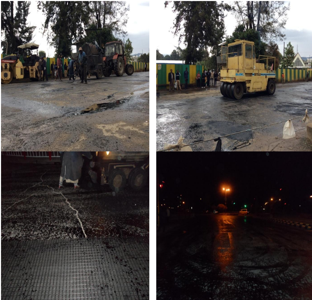
Fig. 3.8: Photo application of tack coat before laying of geogrid at the Gandhi Hospital and National Theatre sites.
