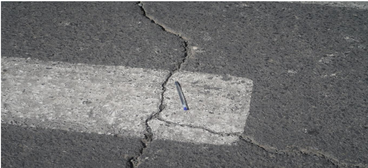
Fig. 4.4: Photo: National Theatre 2 site: Crack before the installation of the Geogrid.
