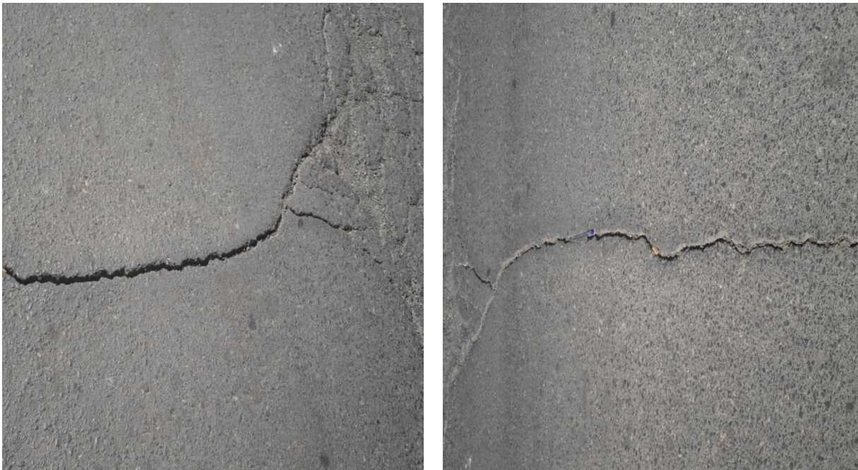
Fig. 3.1: Photos, Reflection cracks at the National Theatre 1 and National Theatre 2
