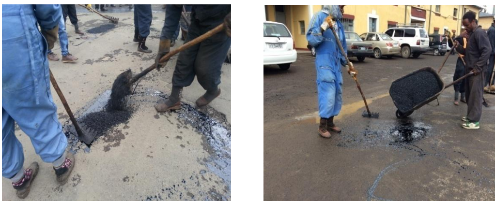
Fig. 3.4: Photo: Application of leveling course to treat potholes and other road defects.
