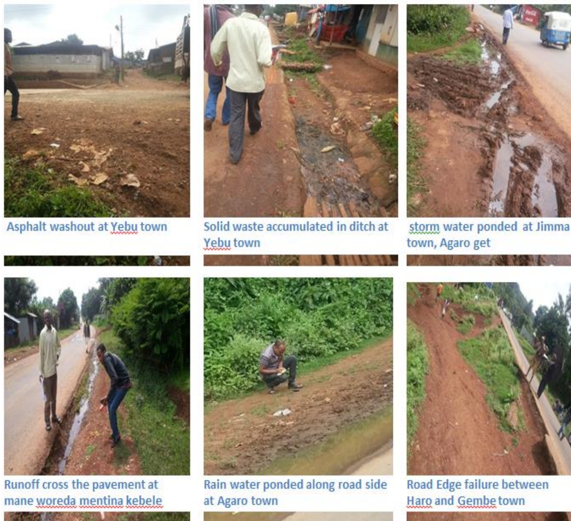
Figure 4.15 Taken June 12 to15/2016 the major flood prone areas along Jimma –Agaro road section
