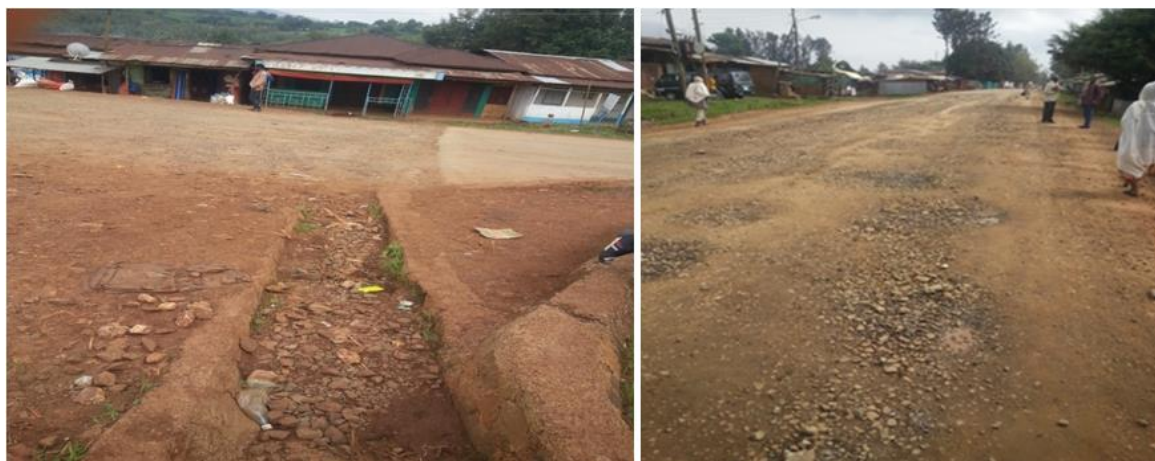
Figure 4.4 Taken august 25/2016 roadside ditches aligned directly to asphalt road at Yebu town.
