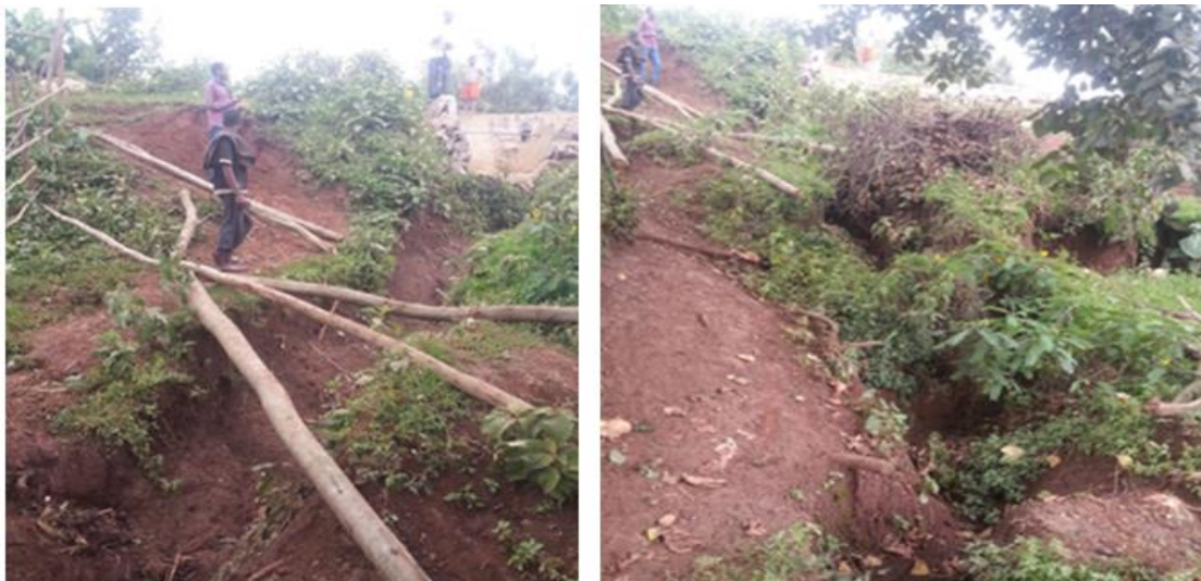
Figure 4.20 problem of roadside drainage outlet at the exit of yebu town
