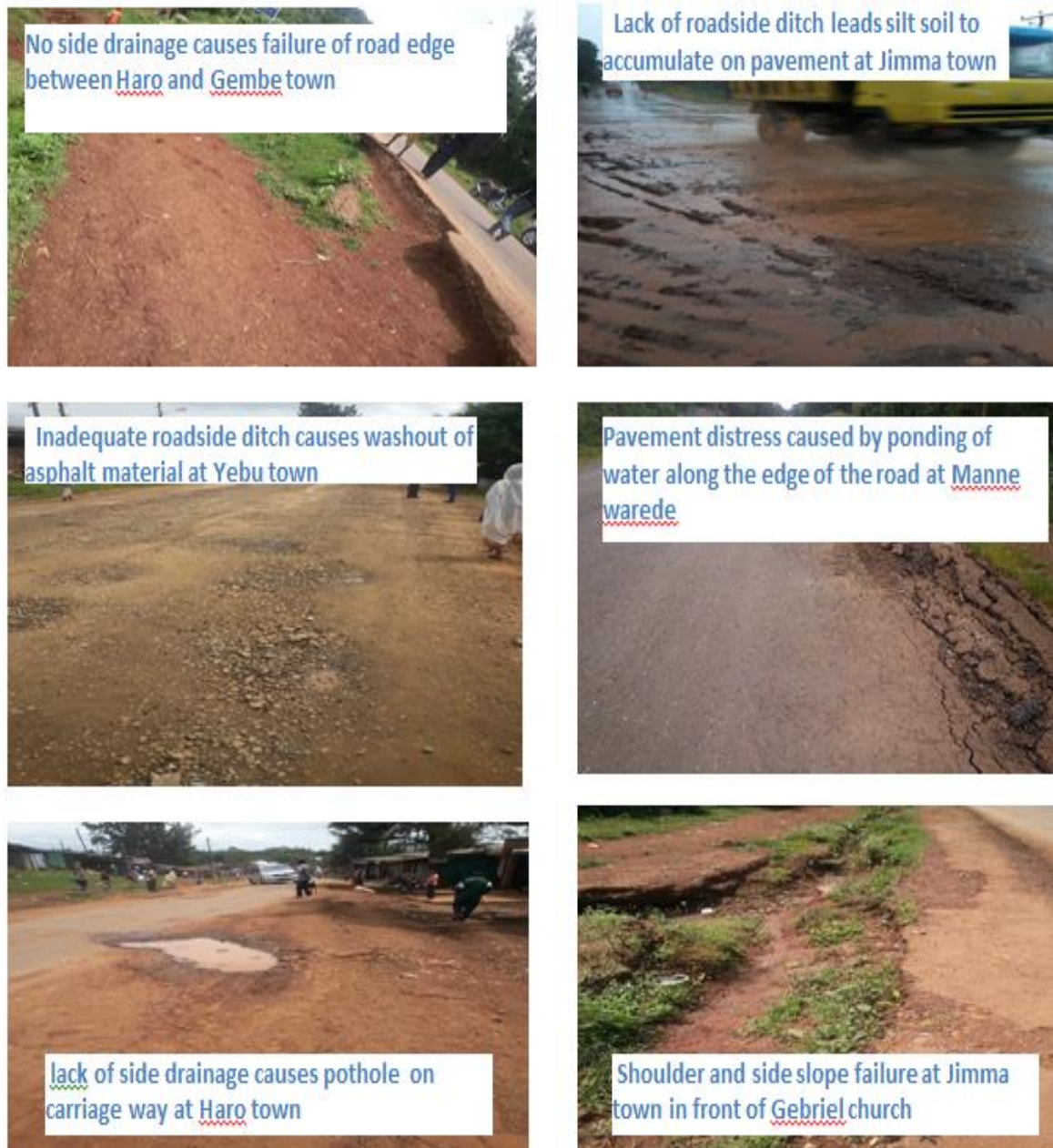
Figure4.17Taken June 12 to 14/2016, Road Surface Damage observed at study area
