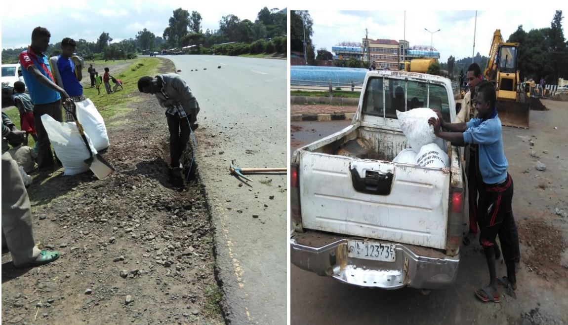
Figure 3-17: Measurement of total depth of excavated pit and transporting it from the stations 13+600-13+800 and 67+926.
