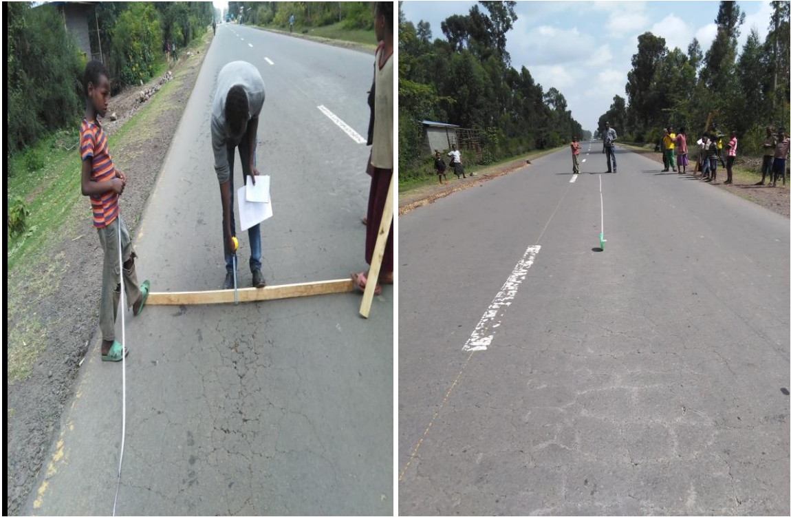
Figure 3-3: Shows the pavement condition surveys on subsection Alaba to Mazoria.
