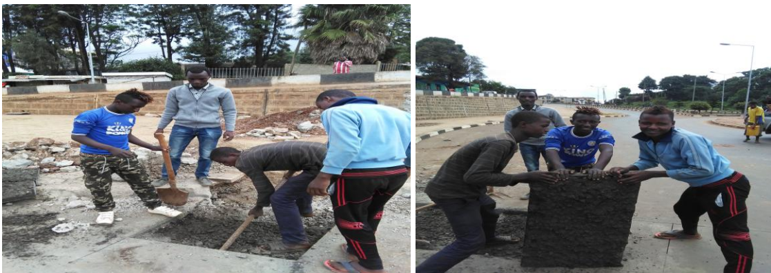
Figure 3-15: Extracting the existing pavement for Sampling of subgrade soil, base course, and sub base materials at Station 67+926 (Sodo Town).
