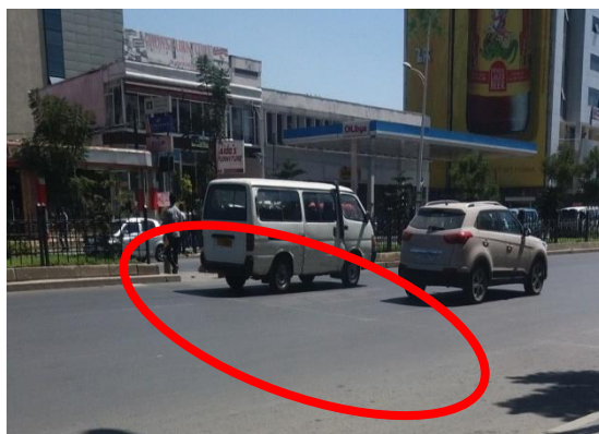
(a) Pedestrian crosswalk not visible
