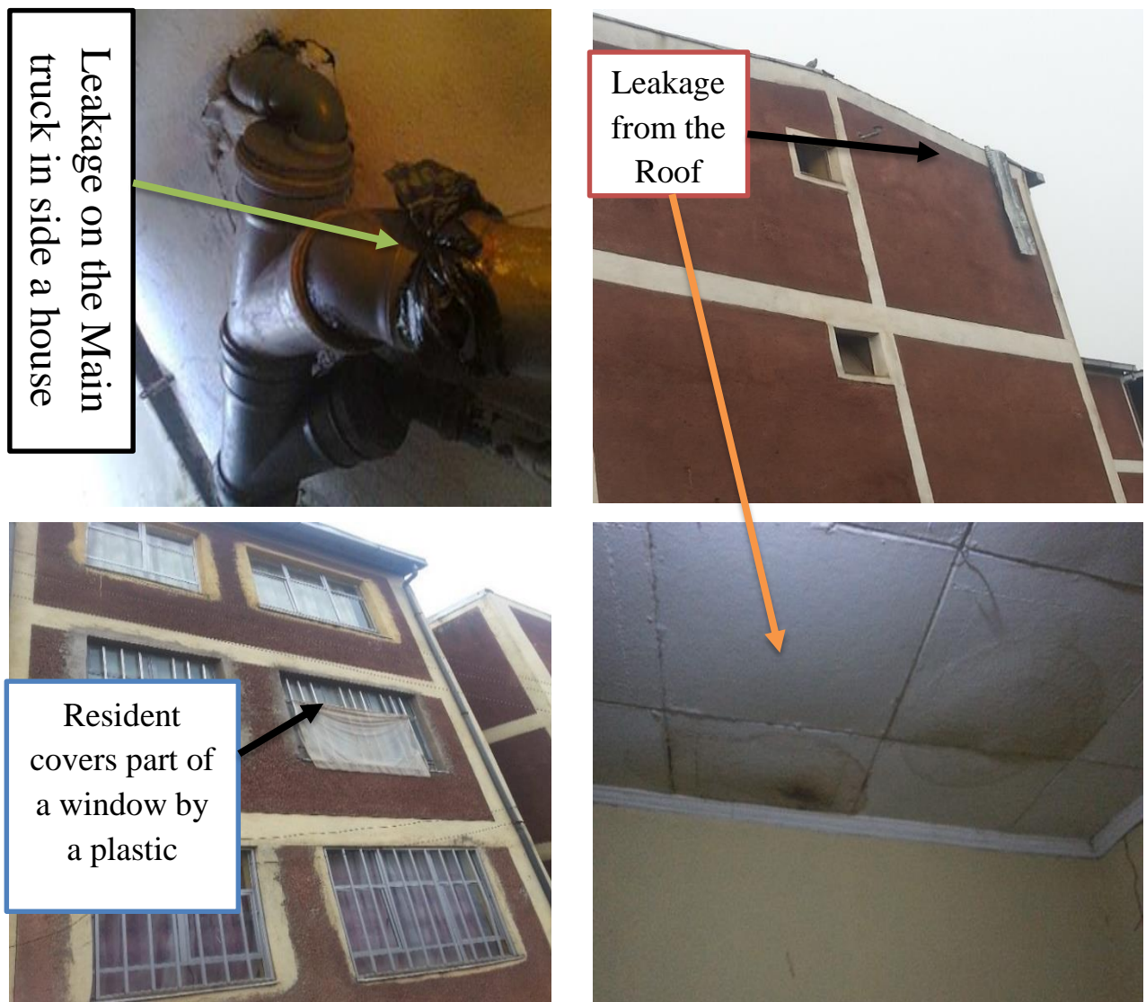
Figure 3. Leakage on different parts of the houses in some selected Blocs/houses in Kella site
