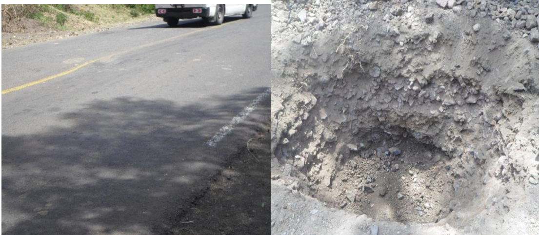
Figure 3.7 Representative Shoved/ Corrugation damaged and their samples (28/09/2008)
