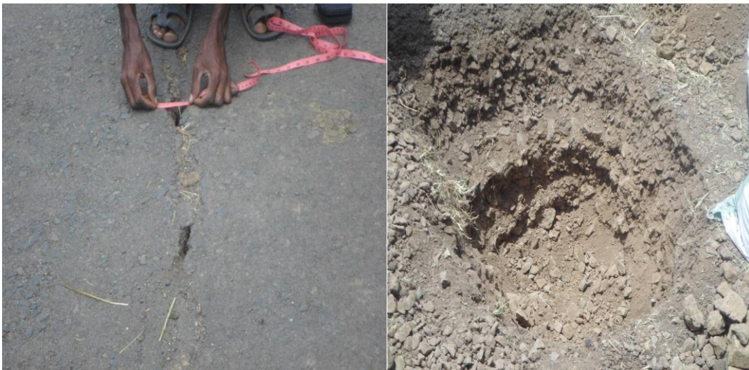
Figure 3.4 Representative Transverse cracks and their sample (20/09/2008)
