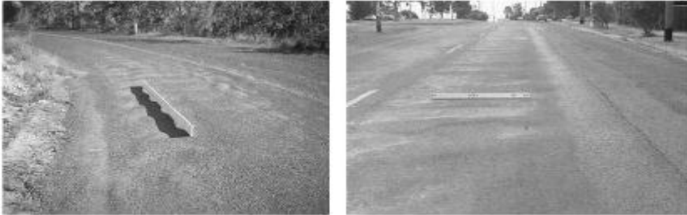
Figure2.2: Corrugations in flexible pavements (Source: Zahidul, 2006).
