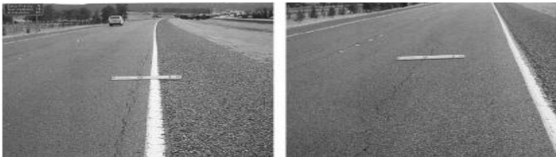
Figure2.7: Longitudinal Cracks in flexible pavements (Source: Zahidul, 2006).
