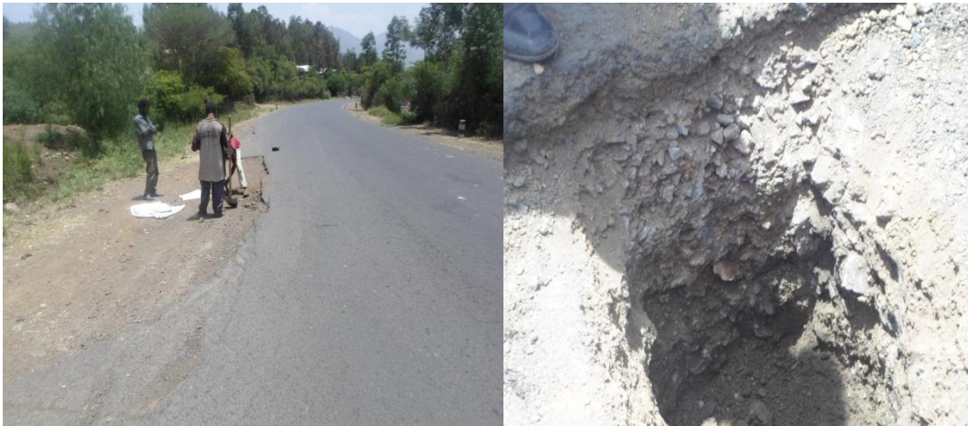
Figure 3.9 Representative Potholes/debonding damages and their samples (29/09/2008)
