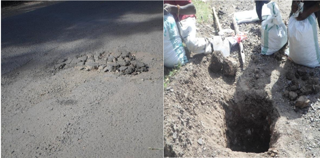
Figure 3.5 Representative patched damaged and their samples (23/09/2008)
