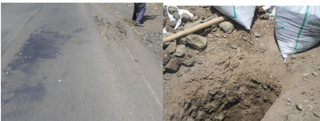
Figure 3.8 Representative Rutting damaged and their samples (28/09/2008)
