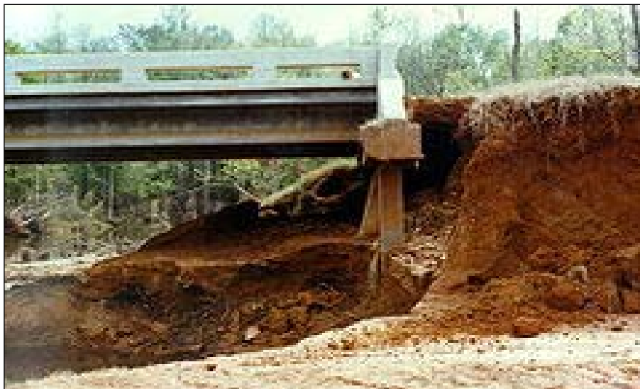
Figure 7: Scouring and Erosion
