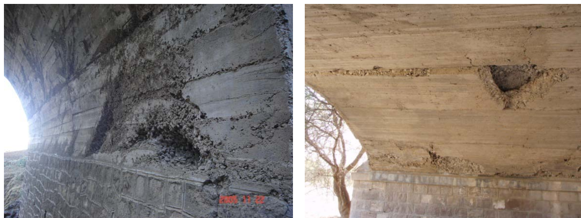
Figure 3: Non Structural crack
