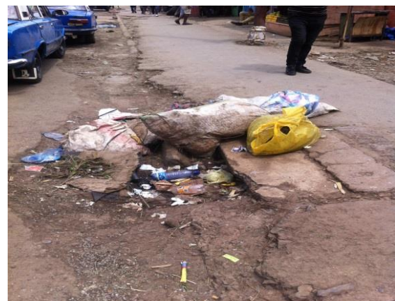
Fig 3.5 f) Curb inlet opening Curb inlets opening blocked by solid waste
