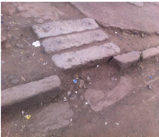
Fig3.5 c) Inlets with cover but totally filled with silt and out of function
