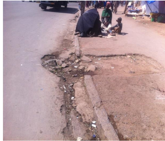
Fig 3.5 b) Inlets without cover (removed), filled with silt and out of function
