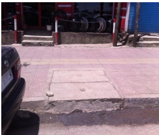
Fig3.5e) Curb inlets opening blocked by cement mortar
