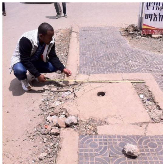
Fig 3.6 e) Curb inlets opening Filled with silt and out of function
