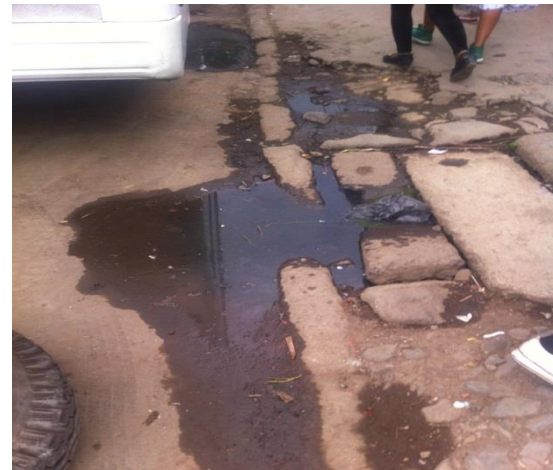
Fig 3.5 d) Inlet operate with problem
