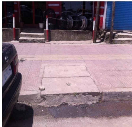
Fig 3.6 f) Curb inlet opening Blocked by cement Mortar
