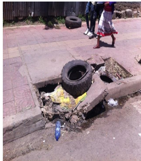
Fig 3.6 b) Inlets without cover (removed), Filled with silt and out of function
