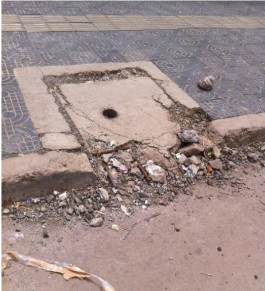
Fig 3.6 c) Inlets with cover but totally filled With silt and out of function
