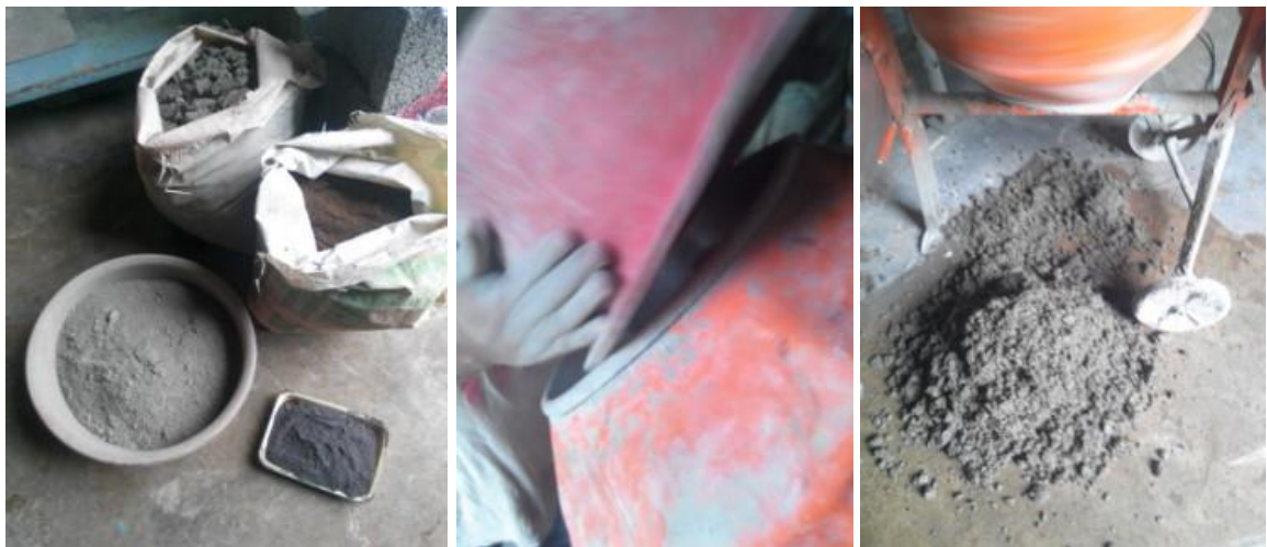
Photo 12 Concrete ingredients to be mixed (left), being mixed (centre) and after mixed (right)
