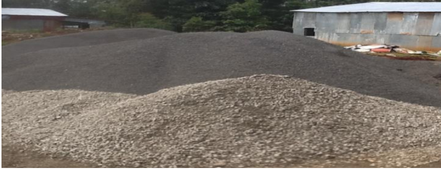
Figure 4-13: Good handling of fine and course aggregates at VARNERO construction project site
