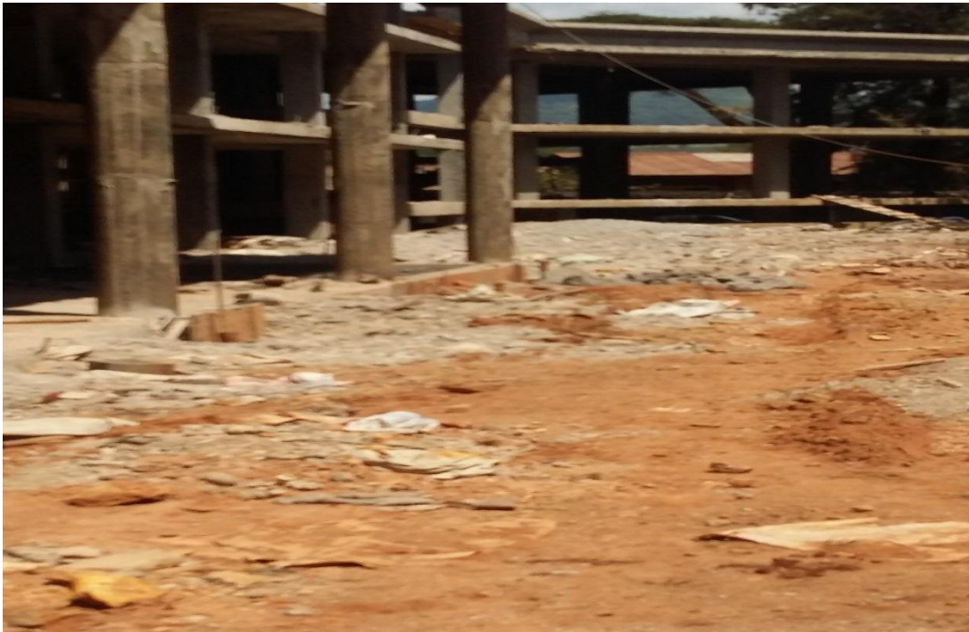
Figure 4-10: Concrete wastage during on construction activities on VARNERO site.
