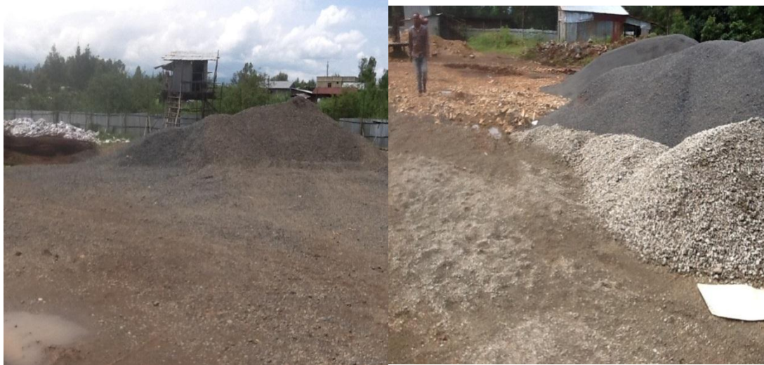
Figure 4-11: Poor handling of premixing concrete at Yotek construction project site
