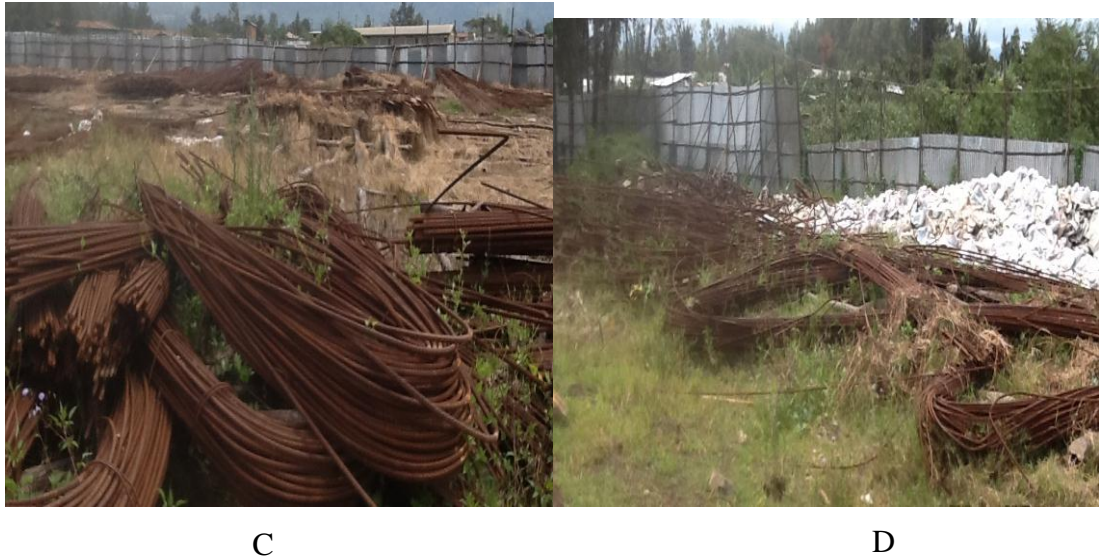
Figure 4-15: Poor Storage and handling of Steel Reinforcement on construction sites
