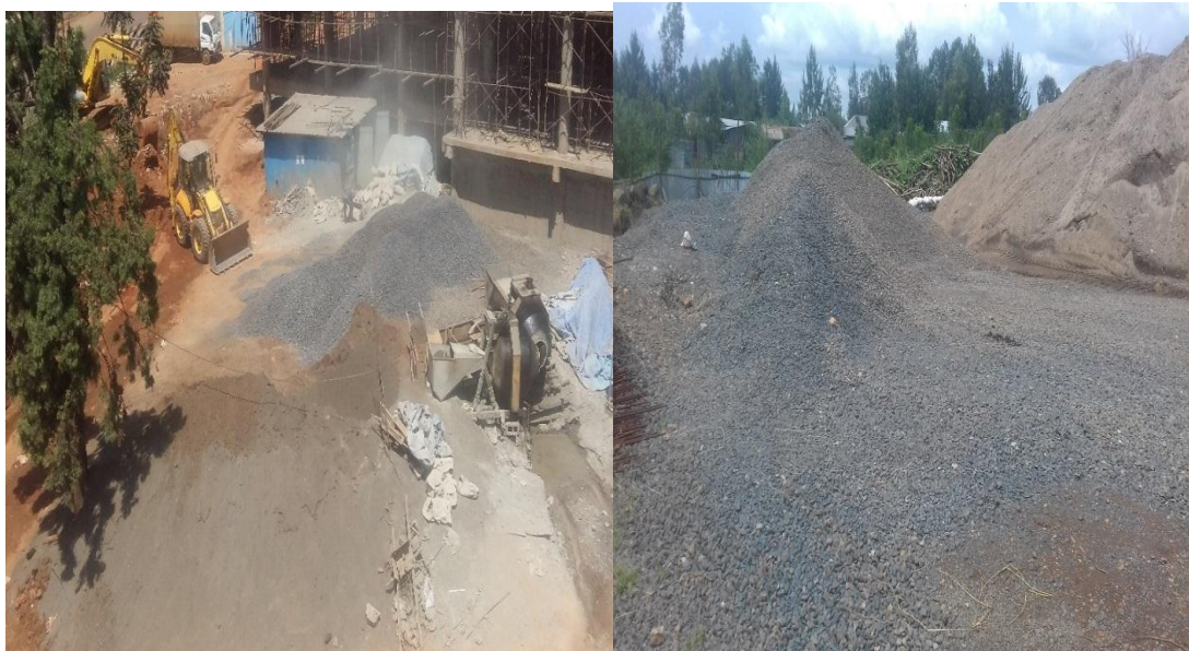
Figure 4-12: Poor handling of fine and coarse aggregates at Yotek construction project site
