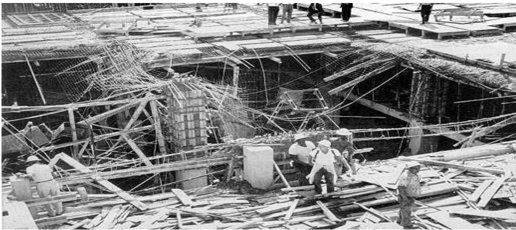
Figure 2.10: Formwork collapse (Attaullah, 2011).
