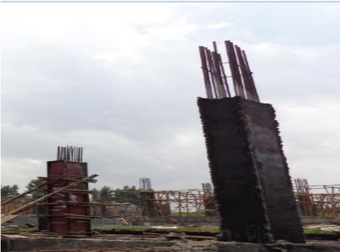
Figure 4.9: Column after stripping of steel formwork some roughness and discoloration on concrete surface at legetafo site.
