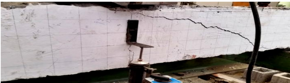
Figure4. 16 Failure mode for TB-4 under cyclic loading
