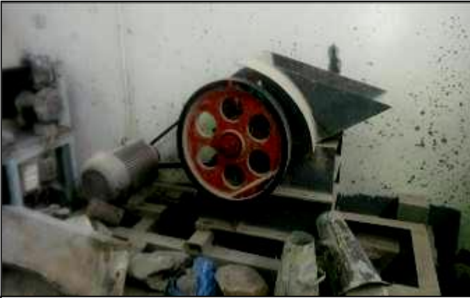
Figure C.1.1: Aggregate Crushing Machine
