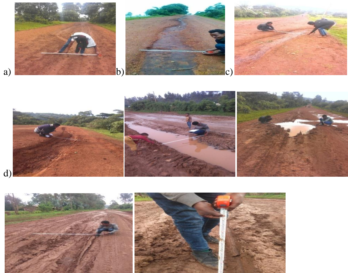
Figure 3.4:A) rutting B) longitudinal erosion, C) and transverse erosion) potholes, distress measurement at different section of the study segment.
