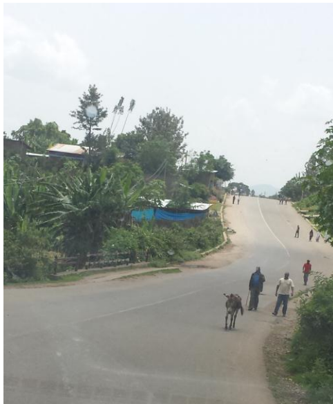
Fig 4.18 no guide post for culvert
