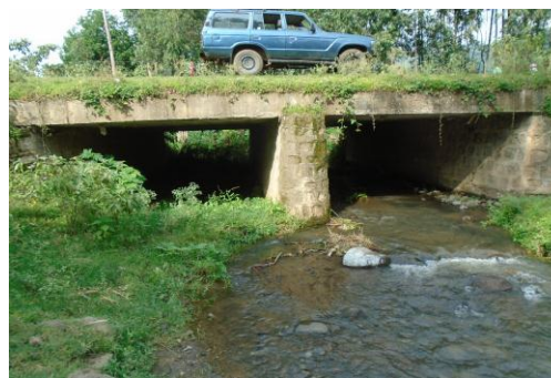
Fig 4.26 Wesha bridge guardrail should be provided
