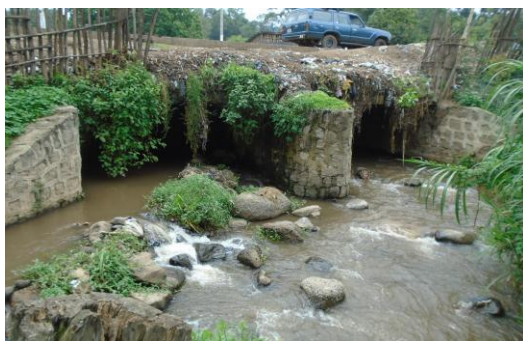
Fig 4.25 Werka Bridge needs maintenance and guardrail should be provided
