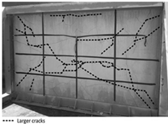
Fig.2.3b. Damaged Wall after blast test [8]
