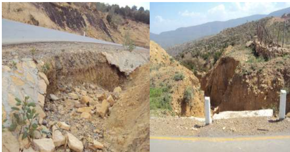
4.4 Figure road side ditches and culverts scouring problems at the study area.
