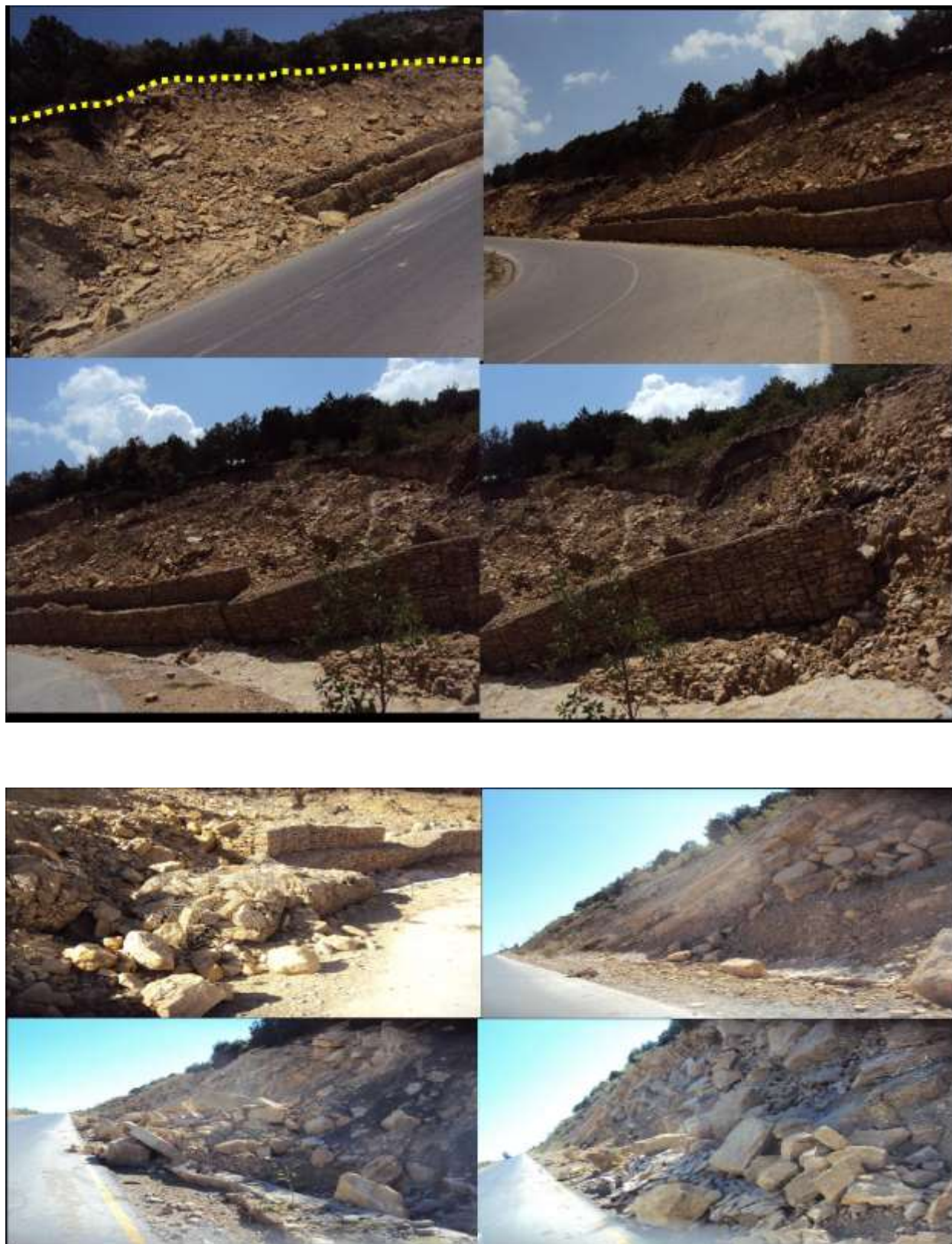
Figure C1.2 Road side ditches scouring problems
