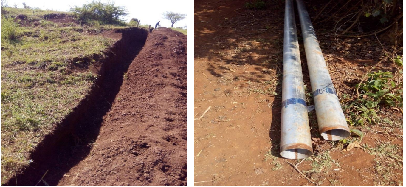
Figure1.7: Duct for pipes and pipes to transport water from Urgessa river to the pond.
