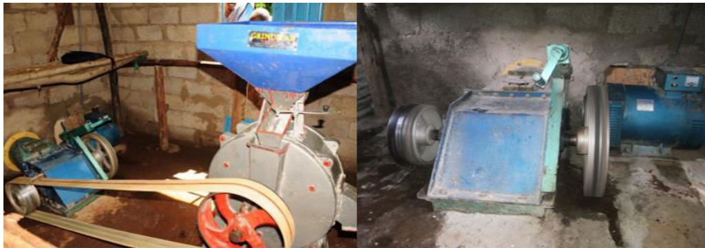
Figure 1.1 Generators of micro hydropower and Water Mill
