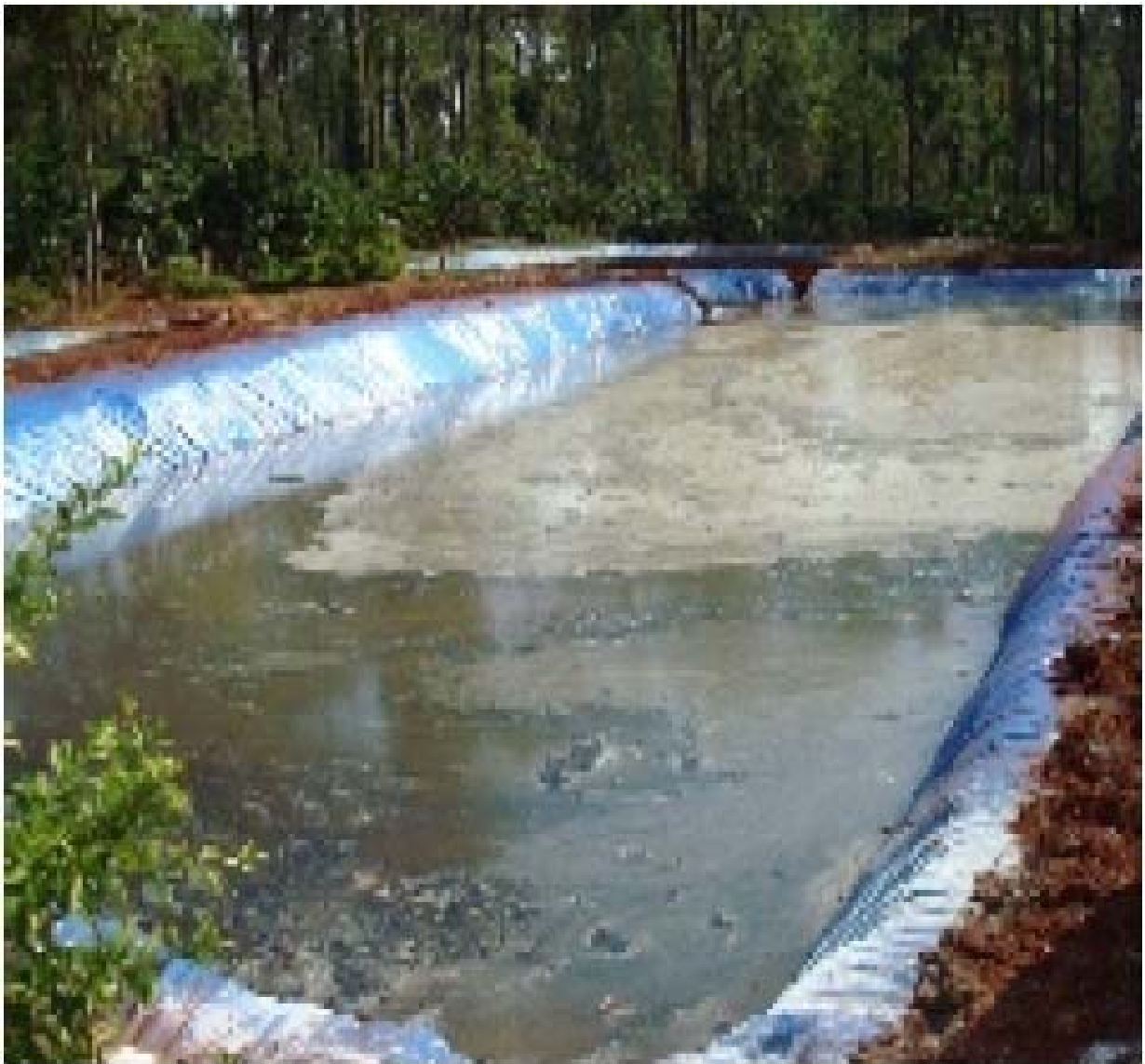
Figure 3. Plastic sheet lined lagoons for treatment of coffee waste effluent
