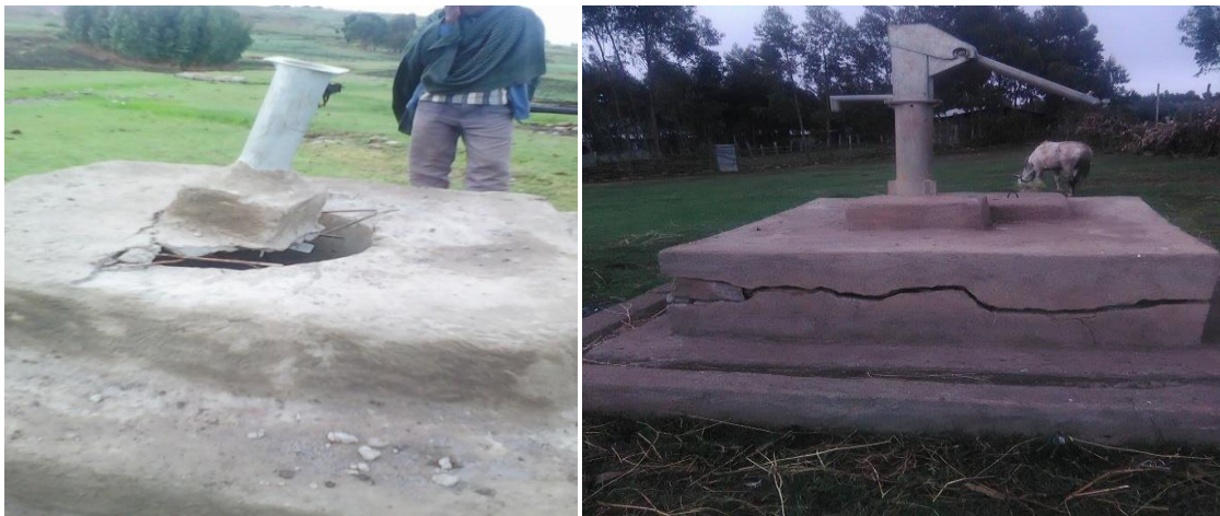
Figure 4: The construction quality of removal of spare parts and cracking of non-functional water supply points in the study area (source: field observation, July 2015)
