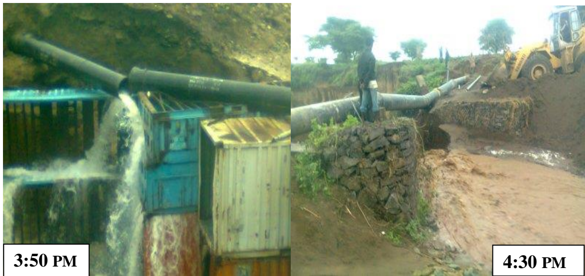
Fig.4. 9 Photo taken during field observation showing problem of fitting and flood hazard
