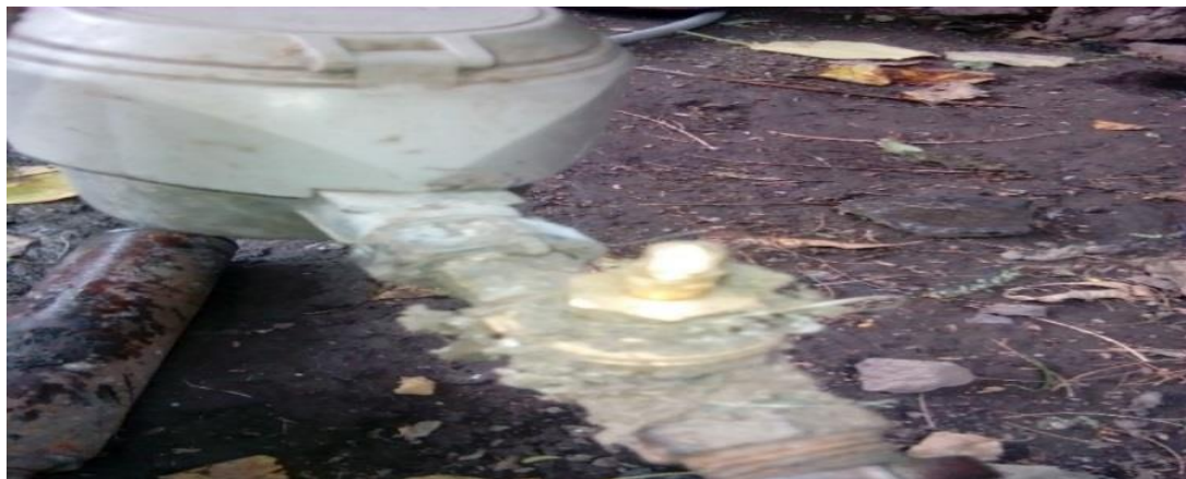
Fig.4. 6 Illegal connection (AWSSE, 2014)
