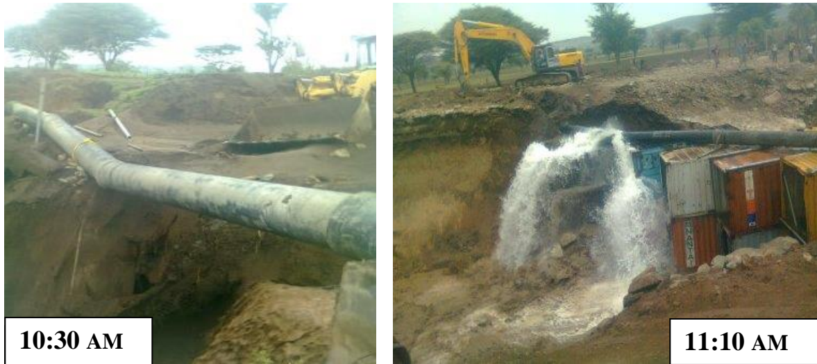
Fig.4. 8 Photo taken during field observation showing poor construction and backfilling
