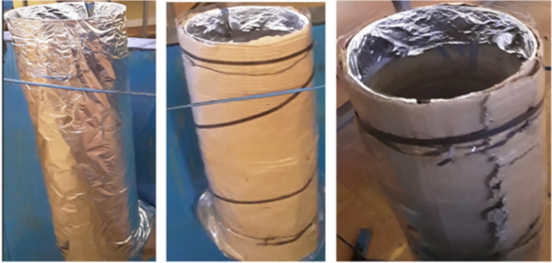
Figure 16: Insulation of heat air conducting tube to minimize heat loss from tube
