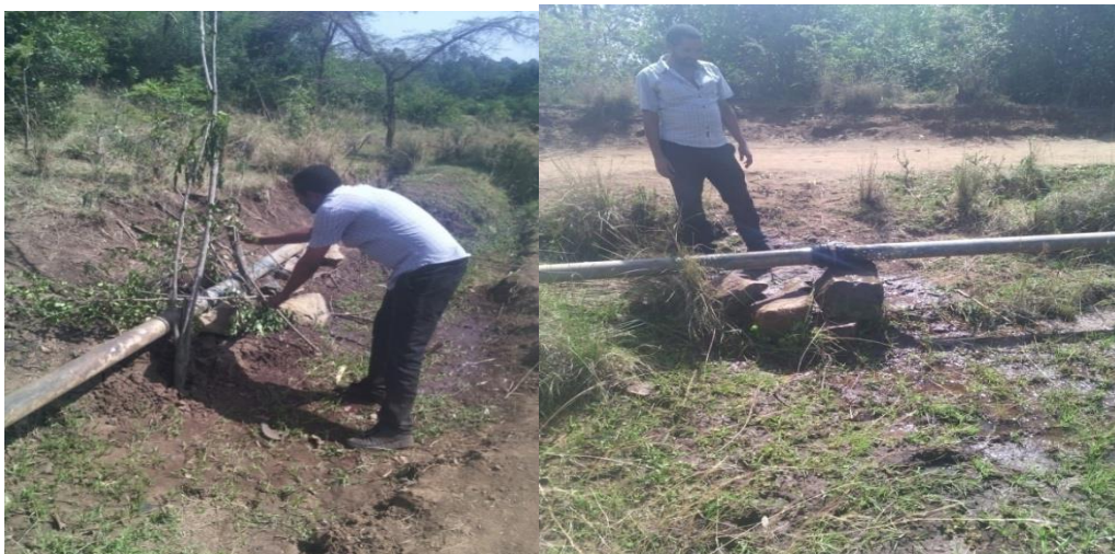
Figure 2 Pipeline design problems in Habicho town
