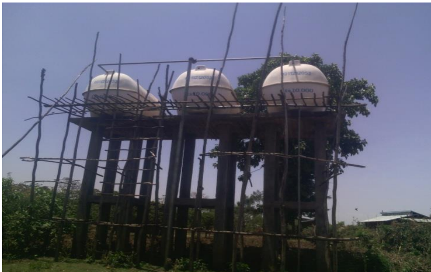
Figure 3 Non-functional overhead tanks in the center of town
