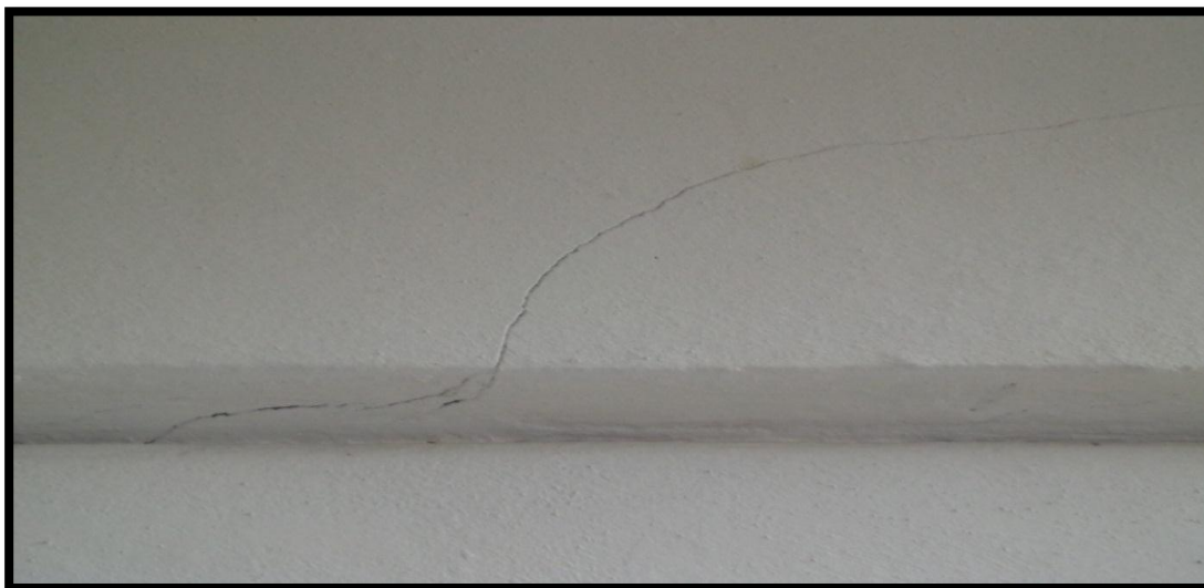
Figure 21 diagonal crack on column from assessed building
