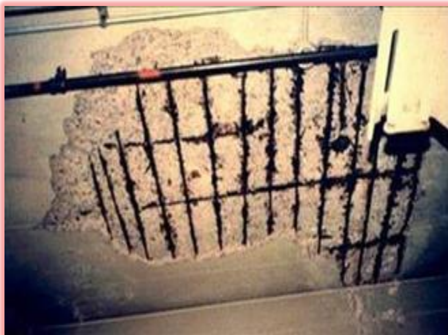
Figure 18 Large spall area [Photo Credit: Robert Pirro]
