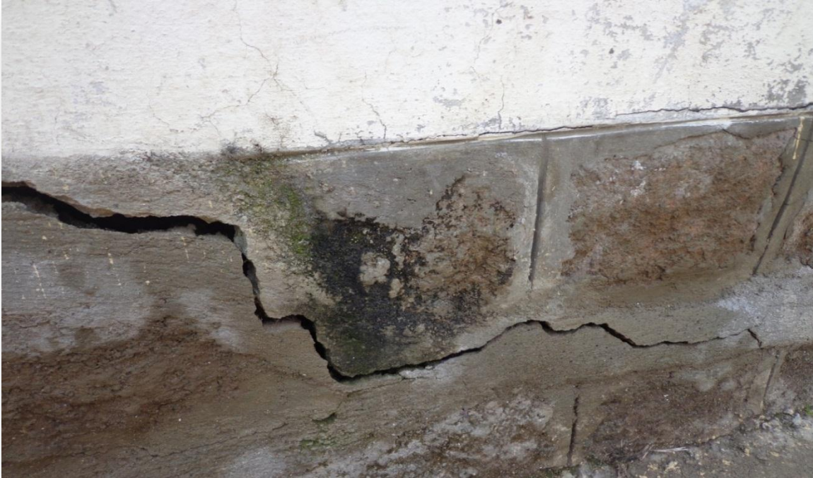
Figure 25 masonry cracking due to foundation settlement from assessed building
