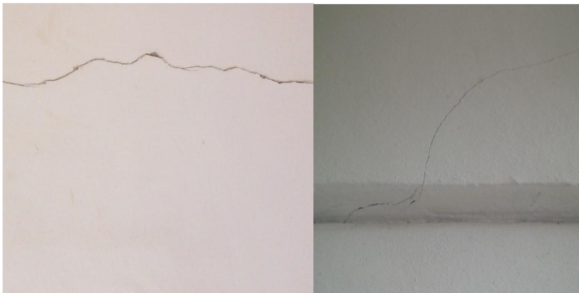
Figure 26 crack width and orientation of the crack
