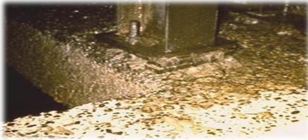
Figure 13 Concrete disintegration around column base [Photo Credit: Robert Pirro]
