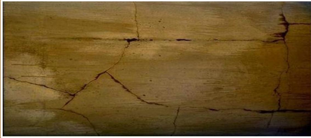
Figure 15 Hardened cracks [Photo Credit: Robert Pirro]
