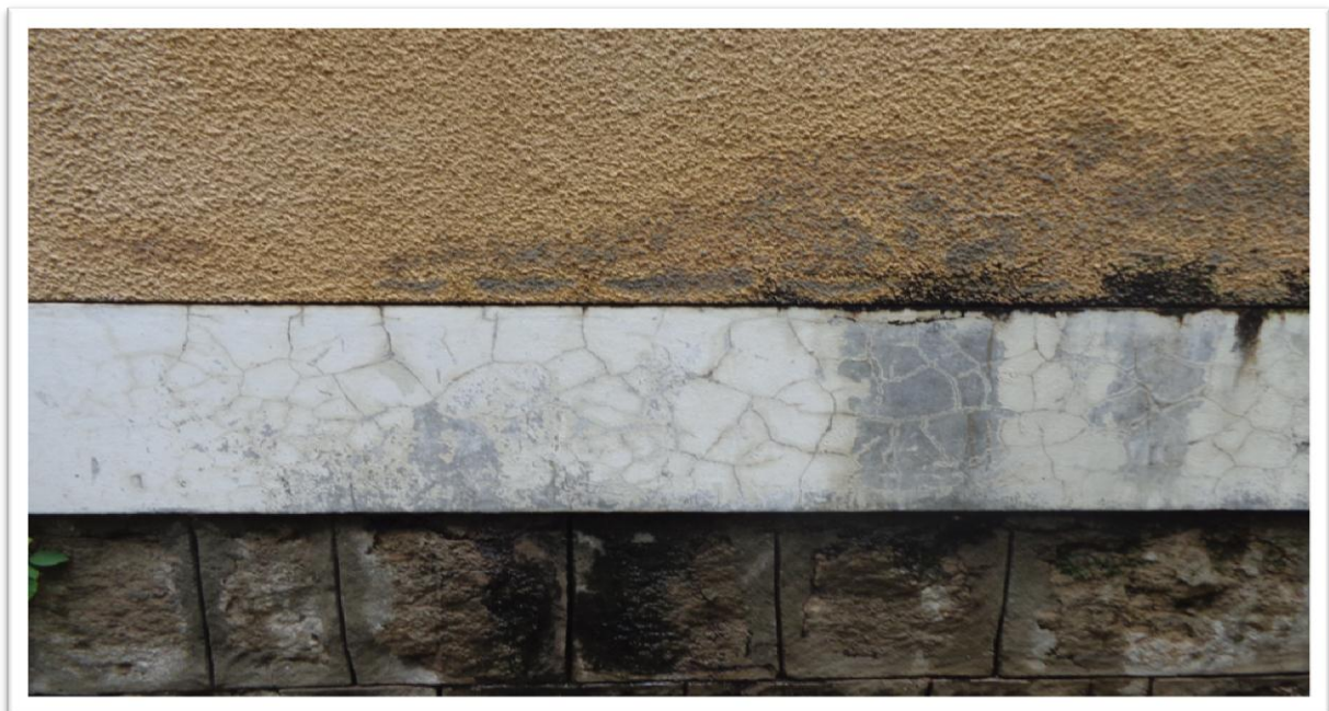
Figure 23 cracks due to water leakages from assessed building
