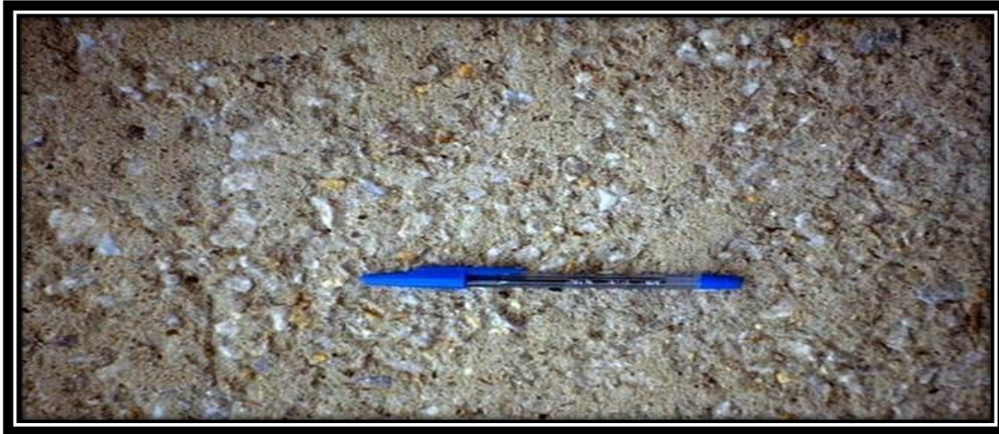
Figure 16 De lamination of concrete caused by premature finishing
