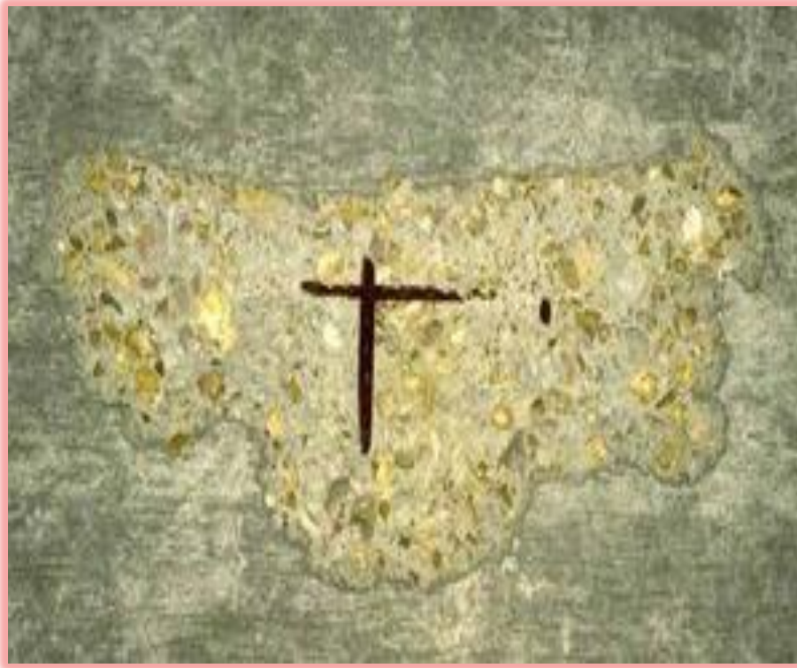
Figure 17 Small spall area caused by corrosion of reinforcement
