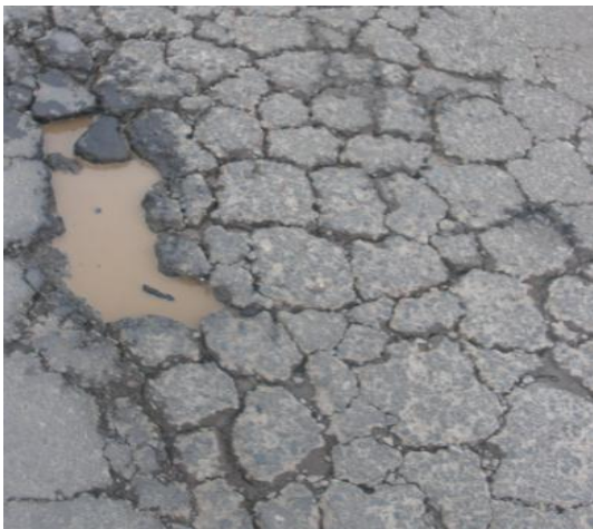
A. Pothole of low severity
