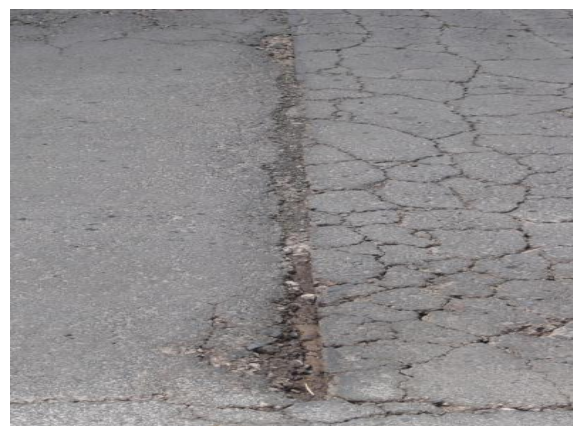
C. Poor Jointing Of Patching
