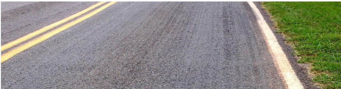
Figure 2.8: Raveling and Pitting
