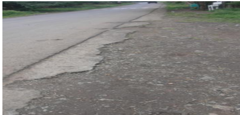
E. Shoulder deformation
