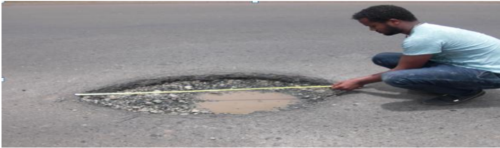
C. Pothole high severity
