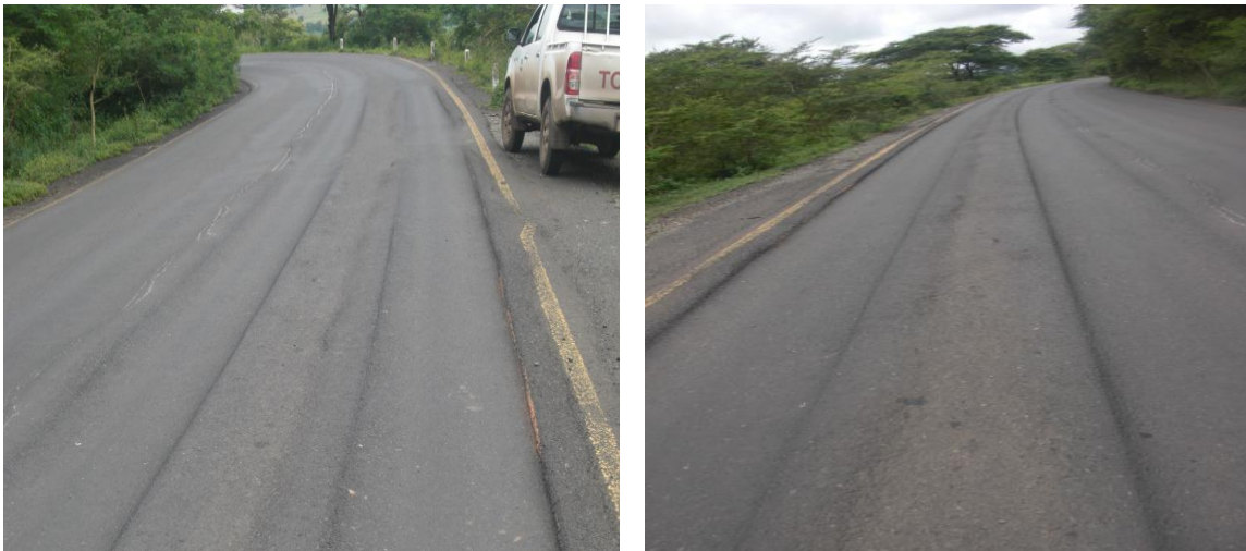
Figure 4.24: Rutting depth 10 cm (High Severity)
