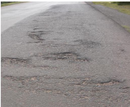
B. Raveling Due To Patching Problem
