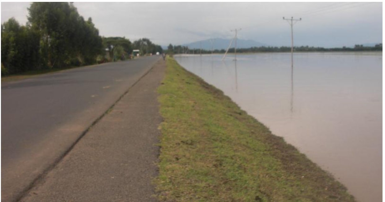
Figure 4.2: High Ponding of Water
