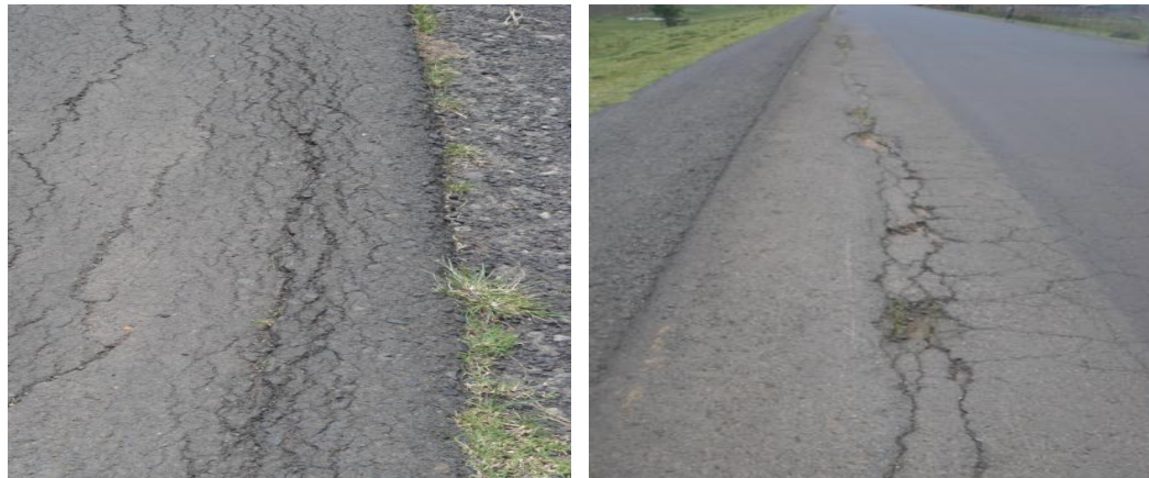
Figure 4.20: Edge/ Corner Crack
