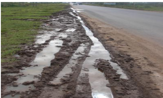
C. Silt- up on shoulder
