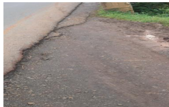
D. Scour on shoulder
