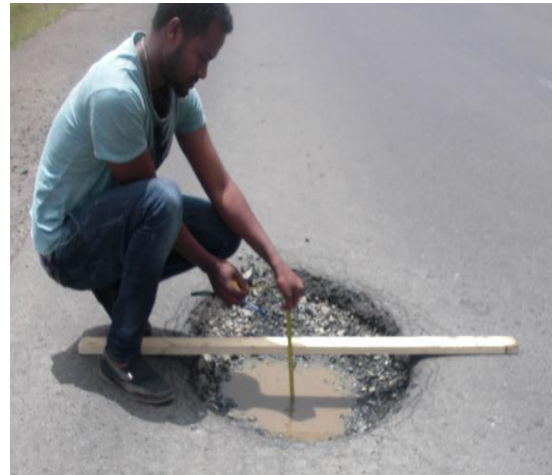
B. Pothole of high severity
