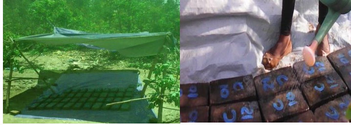
Fig 3.5.3.4.A. Produced bricks in shaded place and curing of bricks by sprinkles of water
