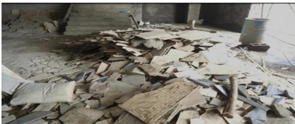
Figure 4.10 Excessive tiles wasted in the construction site.
