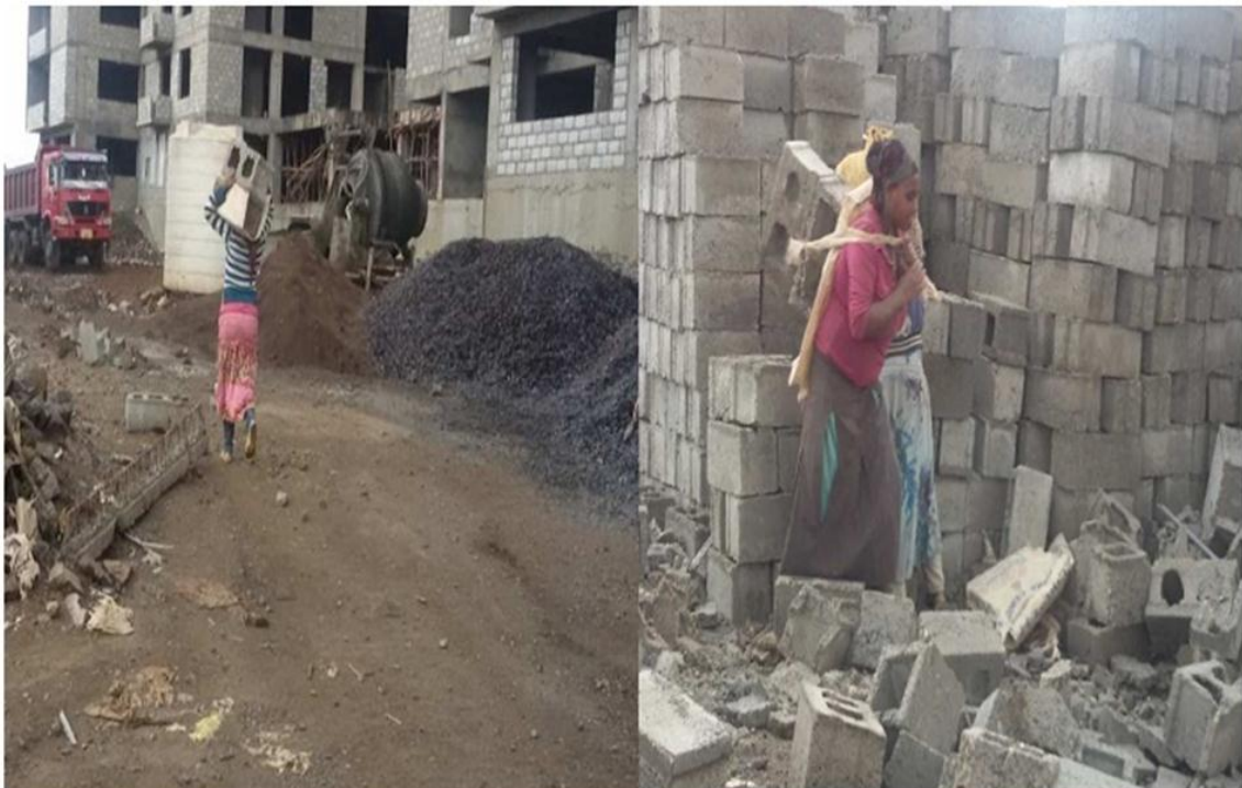
Figure 4.4 Broken concrete hollow blocks due to improper handling on site observed during site visit.
