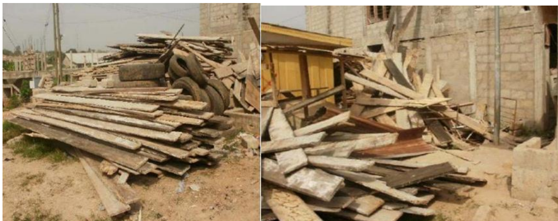
Figure 4.6 Timber form-work poorly stored on site.
