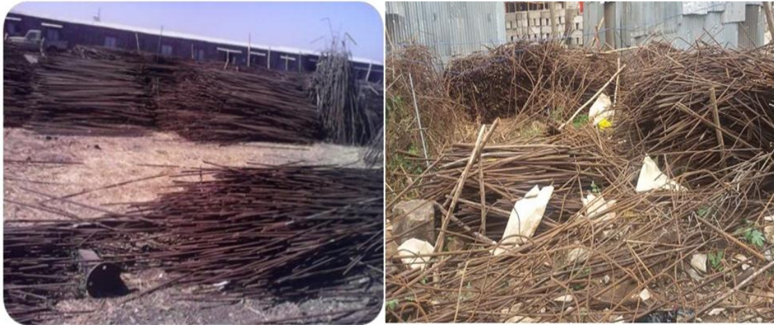
Figure 4.9 wastage of steel reinforcement bar due to Non-optimized cutting and poorly stored on site
