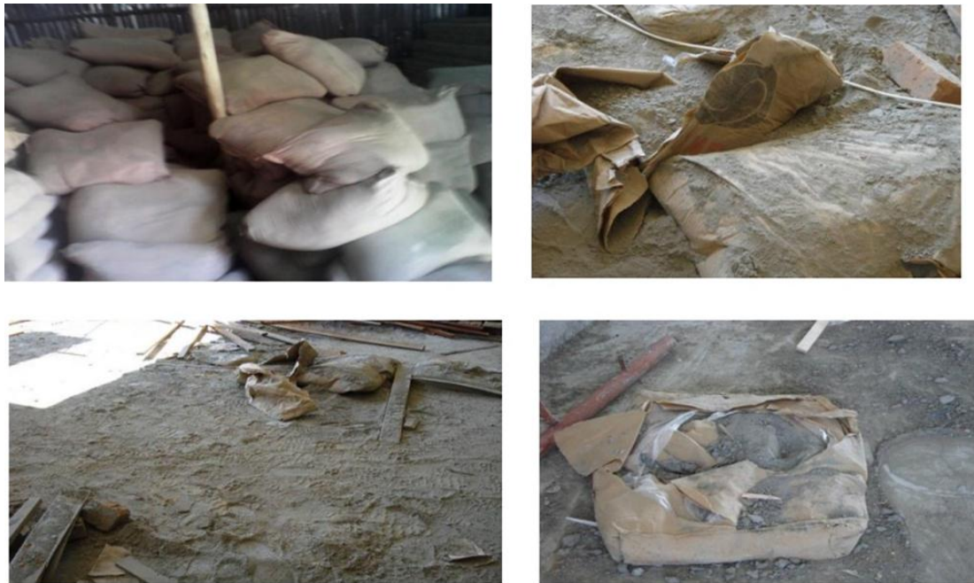
Figure 4.7 improper storage and handling of cement that leads to wastages.
