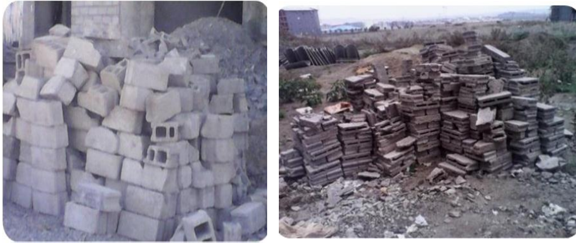
Figure 4.5 shows some of the ways in which blocks are wrongly stored on site.
