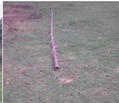
Metal pipe used for distribution of water
