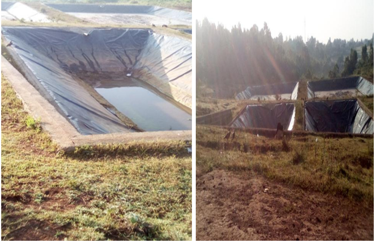
Plates7.. Partial view of the new Built and none Functioning Sanitary Land fill
